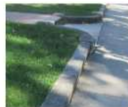
26. Stone curb at the sidewalk edge of Piccadilly St. and Waterloo St.
