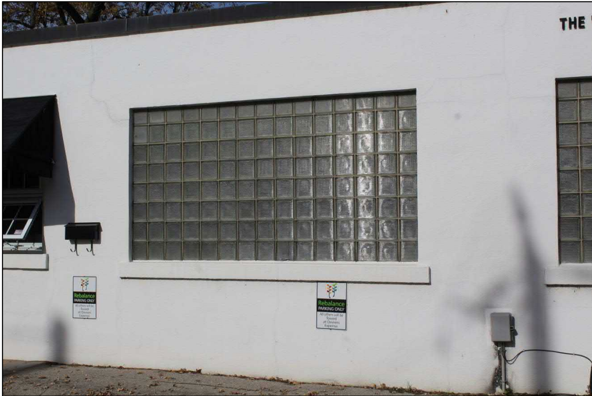
Image 5: Detail of glass block window and concrete window sill, south façade. (AECOM, 2018)
