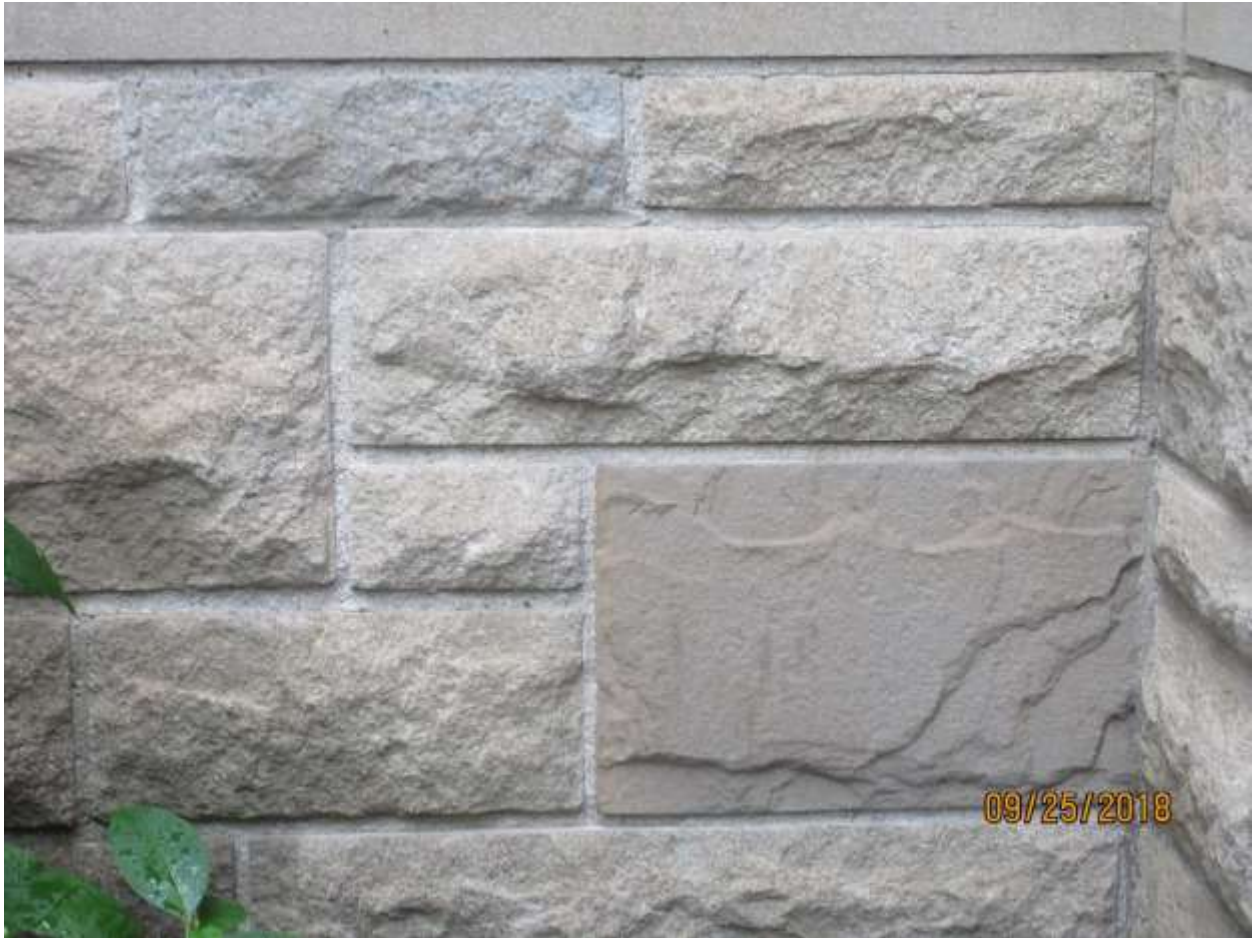
Image 9: Detail of the stone masonry base of the existing built heritage resource at 550 Dufferin Avenue.
