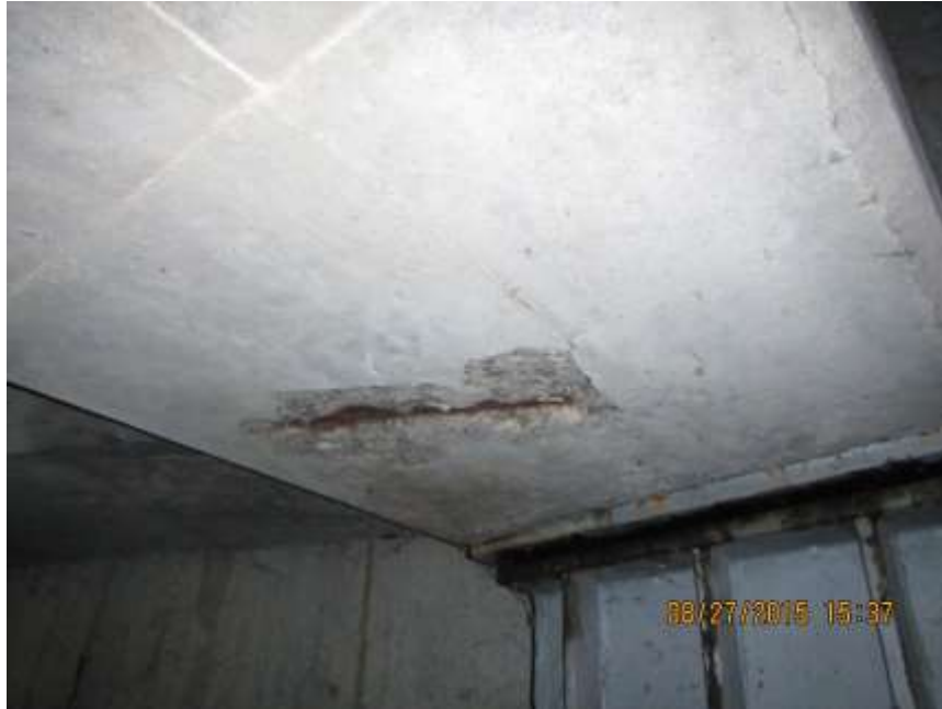
SPALL AT BOTTOM OF GIRDER - AUG'15
