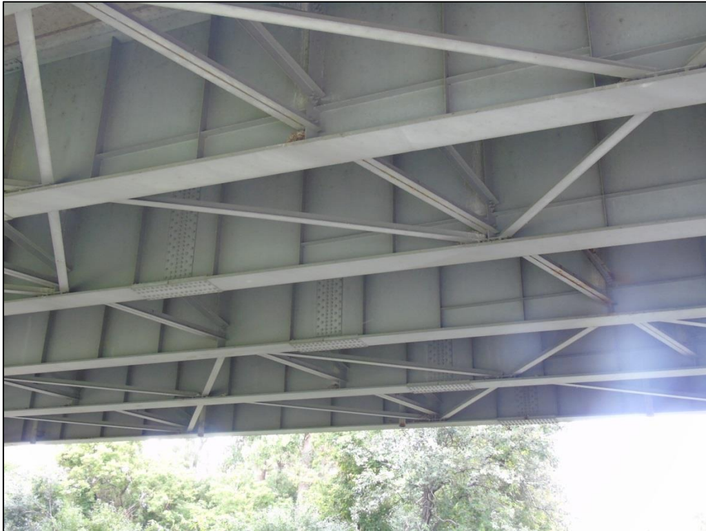
Photograph 20: View showing welded steel plate girders, cross and lateral bracing and bolted gusset plates
