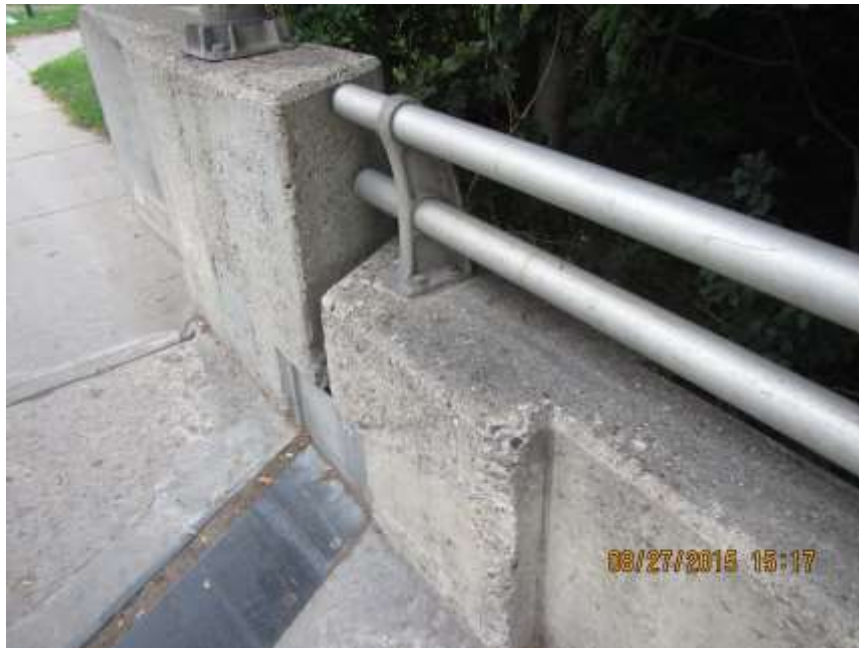
SCALING ON PARAPET WALL - AUG'15
