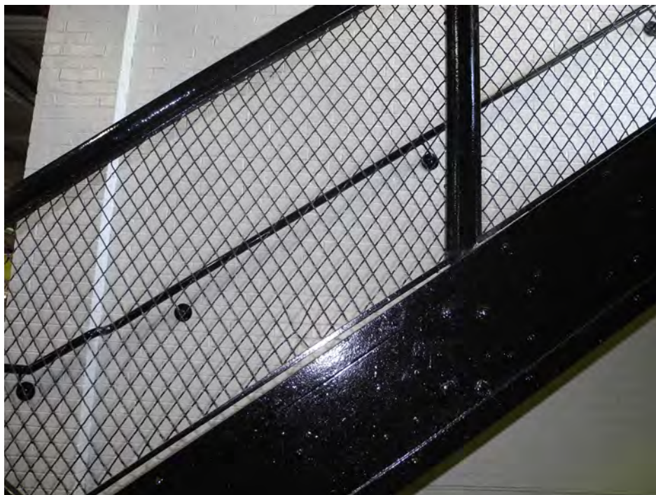
Figure 36 - Industrial metal finishes seen on the eastern stairwell of the Confederation Building, typical throughout (CBCollective 2018).
