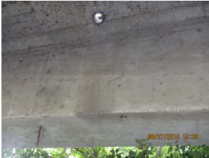
DELAMINATION ON GIRDER - AUG'15
