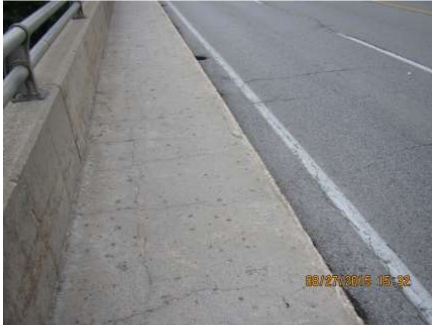
CRACKING AT SIDEWALK - AUG'15
