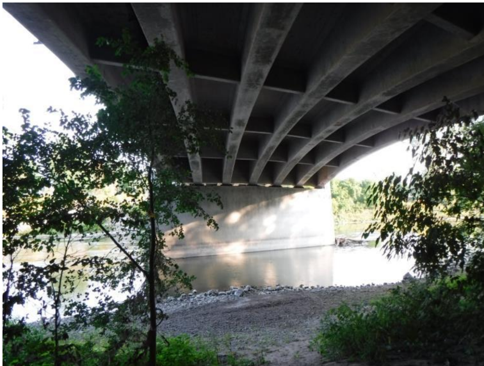
Plate 20: View of the south face of the centre pier. Note the slight skew of the pier.
