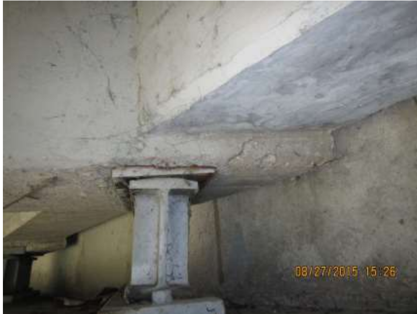
CRACKING AT GIRDER ENDS - AUG'15
