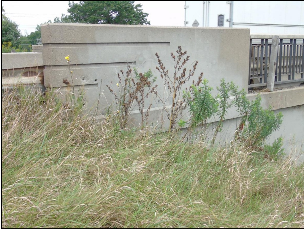
Photograph 22: Concrete end post with horizontal grooves, common for early and mid-20th century bridges
