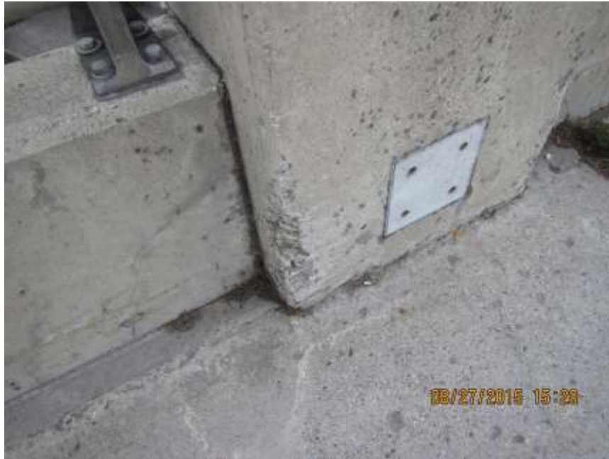
ABRASION AT PARAPET POST - AUG'15
