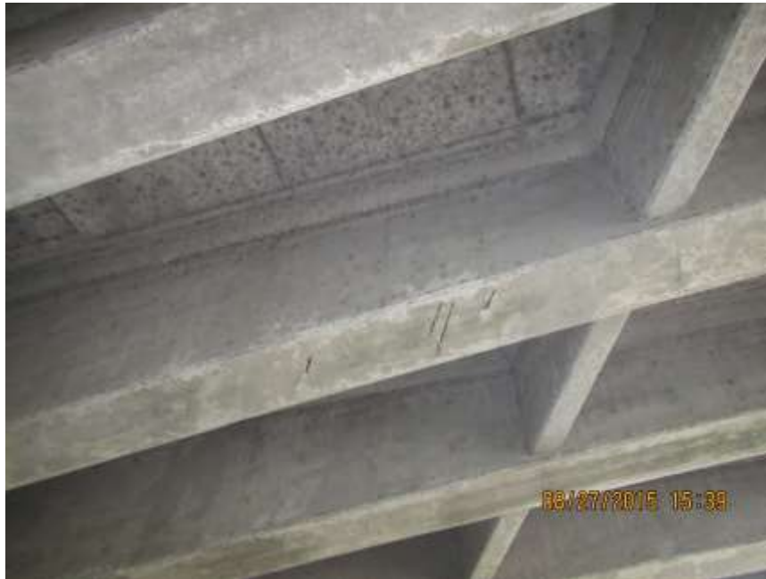
EXPOSED BARS ON GIRDERS - AUG'15
