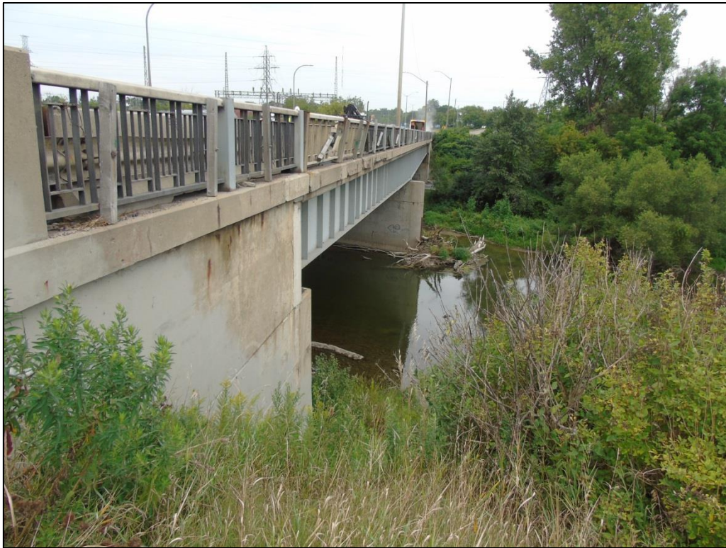
Photograph 6: View showing east side of the bridge and its setting above the Thames River
