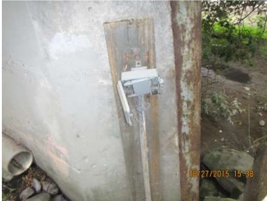
BROKEN ELECTRICAL BOX ON SOUTH PIER - AUG'15
