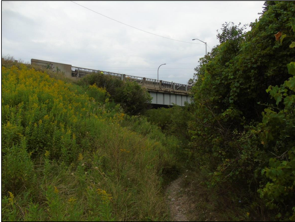
Photograph 12: View looking west showing informal trail that approaches on the south side of the river as it approaches the bridge
