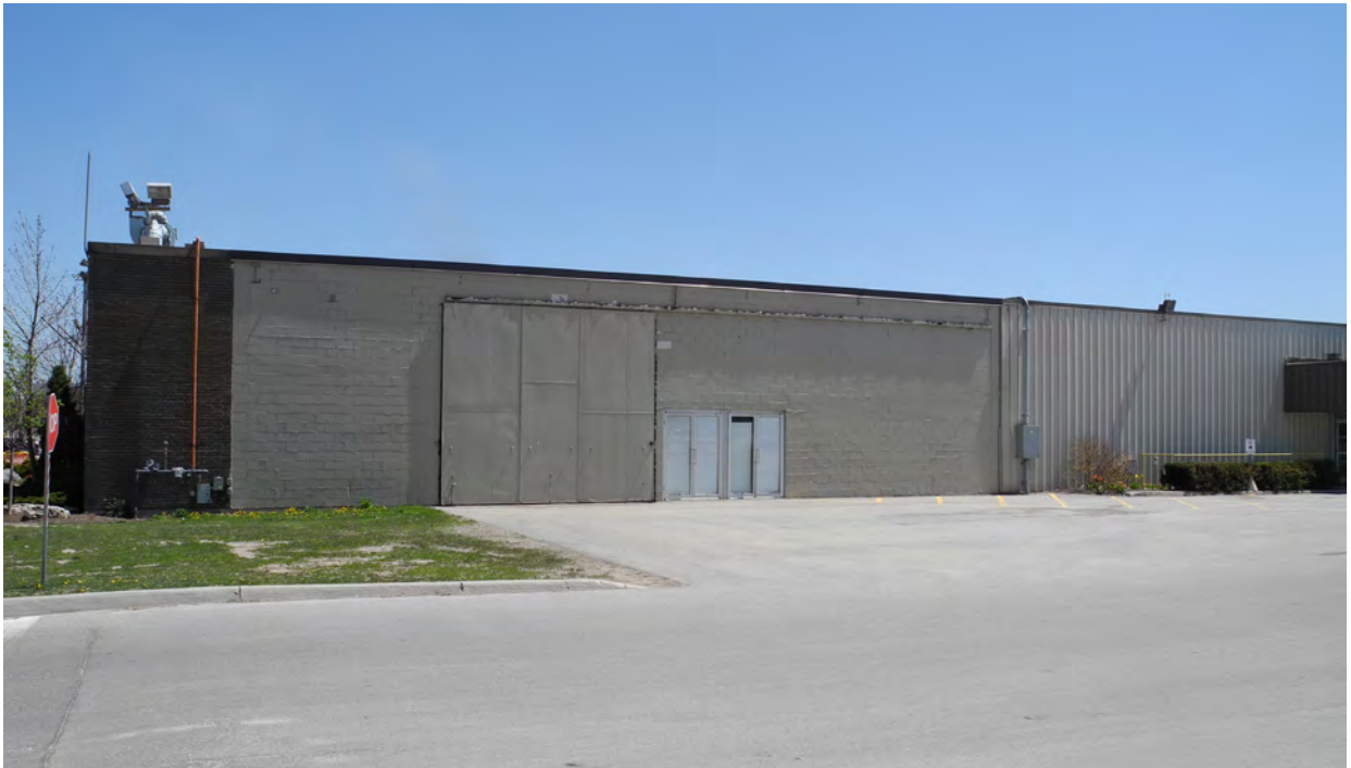
Figure 47 - Scarring and sliding door on the west wall of the Canada Building indicate where the Link connected it with the Poultry Building until 2013 (CBCollective 2018).
