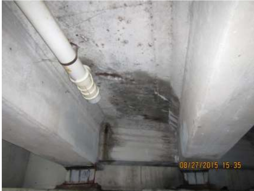
STAINING ON SOFFIT AT SOUTHEAST CORNER - AUG'15
