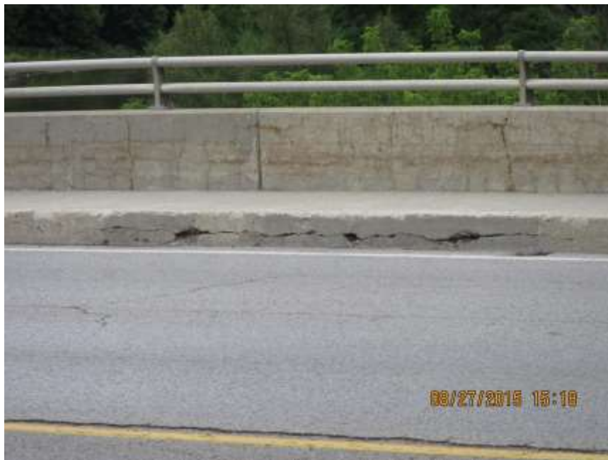
CRACKING AT CURB - AUG'15
