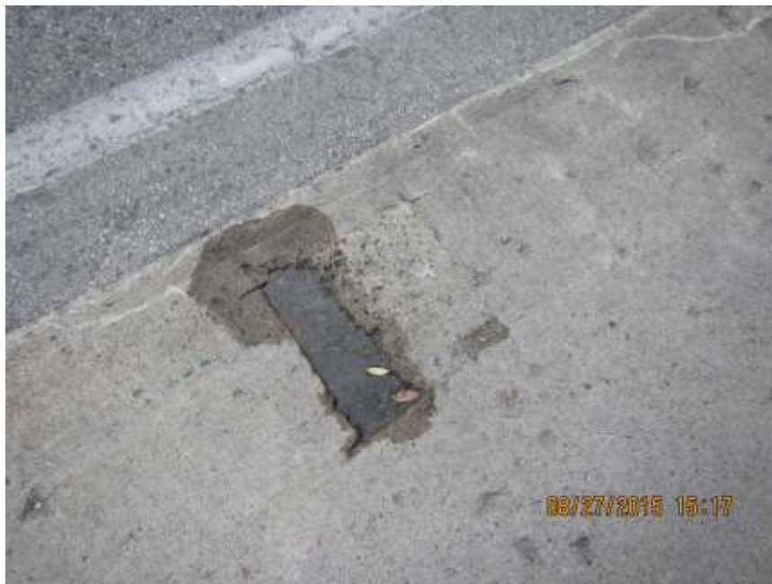
SPALL IN SIDEWALK - AUG'15
