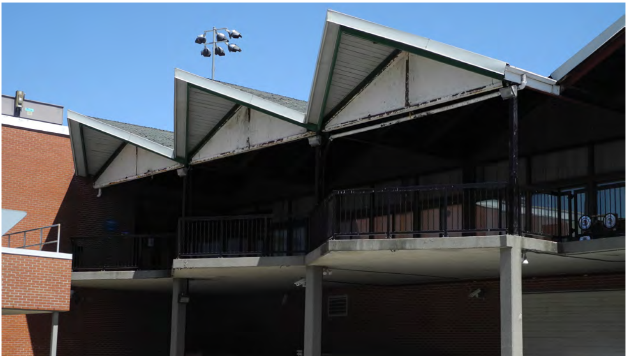
Figure 54 - Modernist detailing on an outdoor area on the Carousel Room's north elevation (CBCollective 2018).
