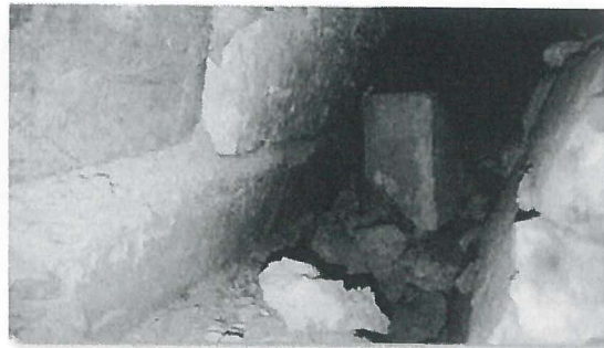
Image 4: Penetration in Exterior Brick Wall at base.
