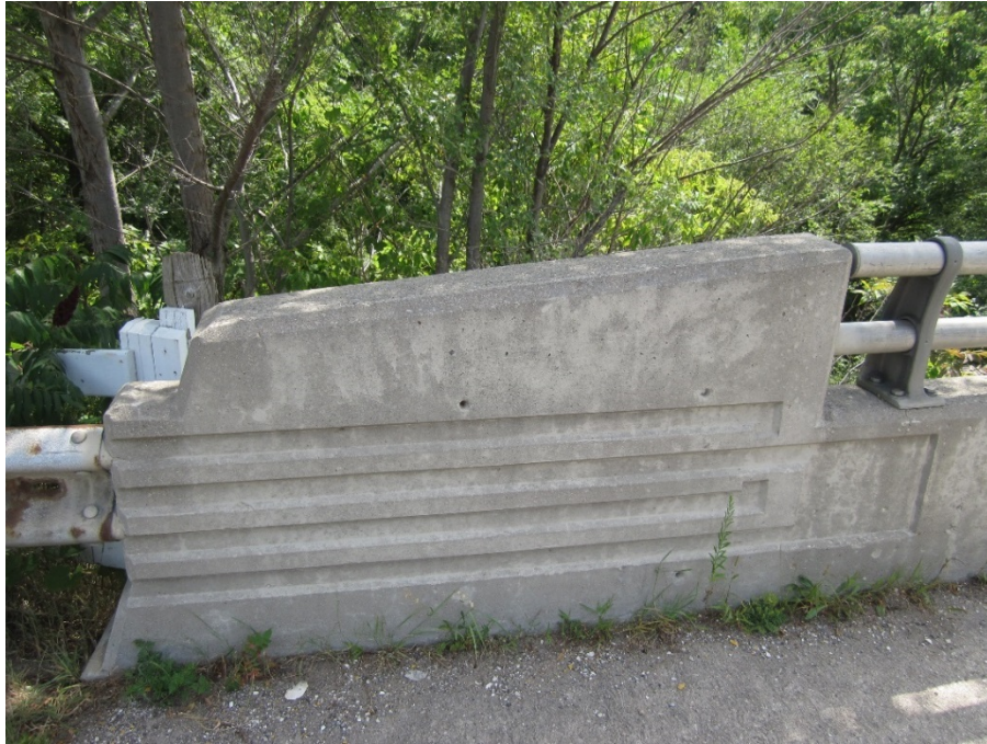
Plate 15: Detail view of the decorative concrete impression at the end railing post
