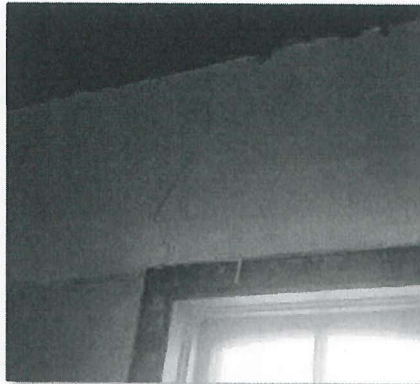
Image 29: Cracking at Window
