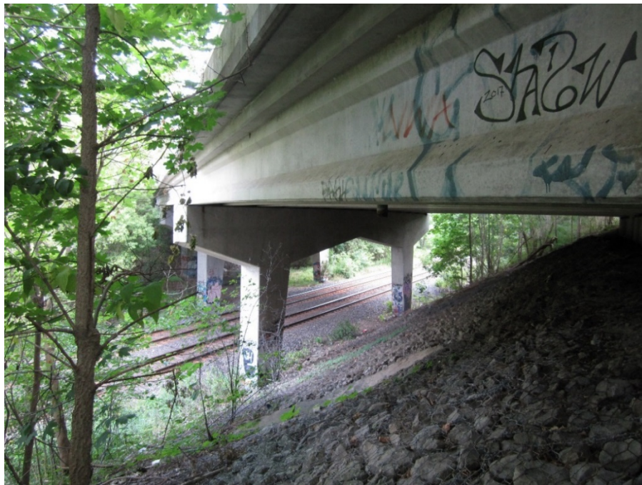
Plate 11: View looking northeast beneath the bridge towards the cast in place concrete piers
