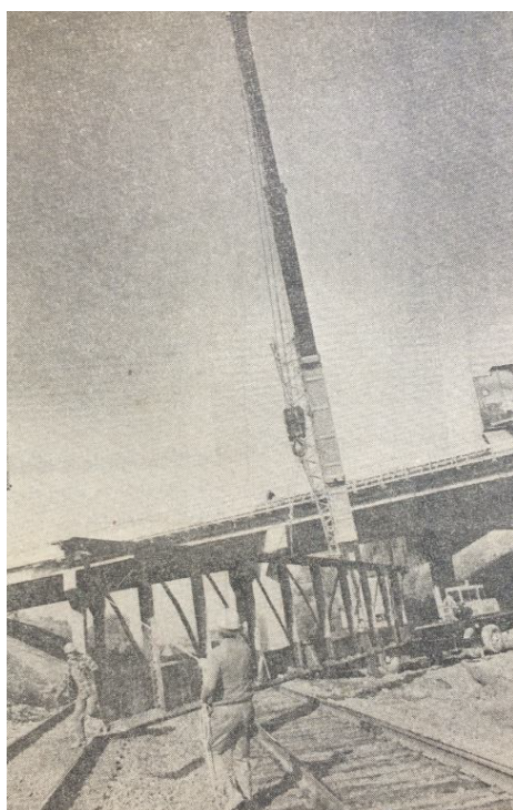
Plate 3: Construction crews remove the steelwork of the old Riverside Bridge, October 1974 (London Free Press, October 9, 1974)
