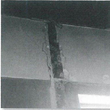
Image 28: Cracking at Window
