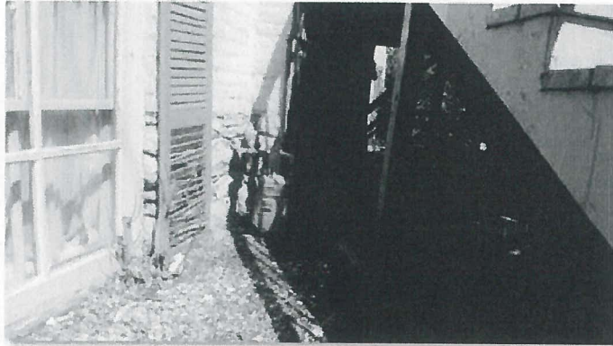
Image 1: West side of exterior wall at main entrance. (Image shows window at grade; Gas Meter Location, Entrance patio framing.)
