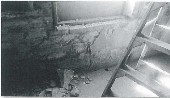
Image 26: Cracked Brick wall at Window
