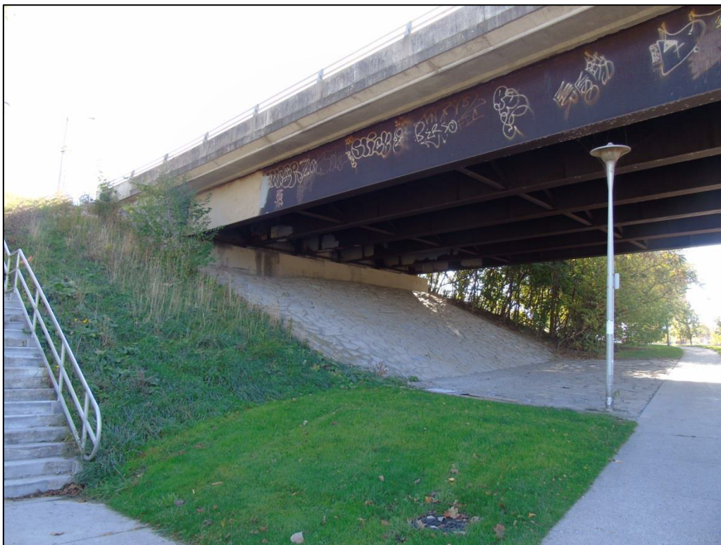
Image 17: East abutment, showing sloping flagstone, and stairway from Queens Avenue at left
