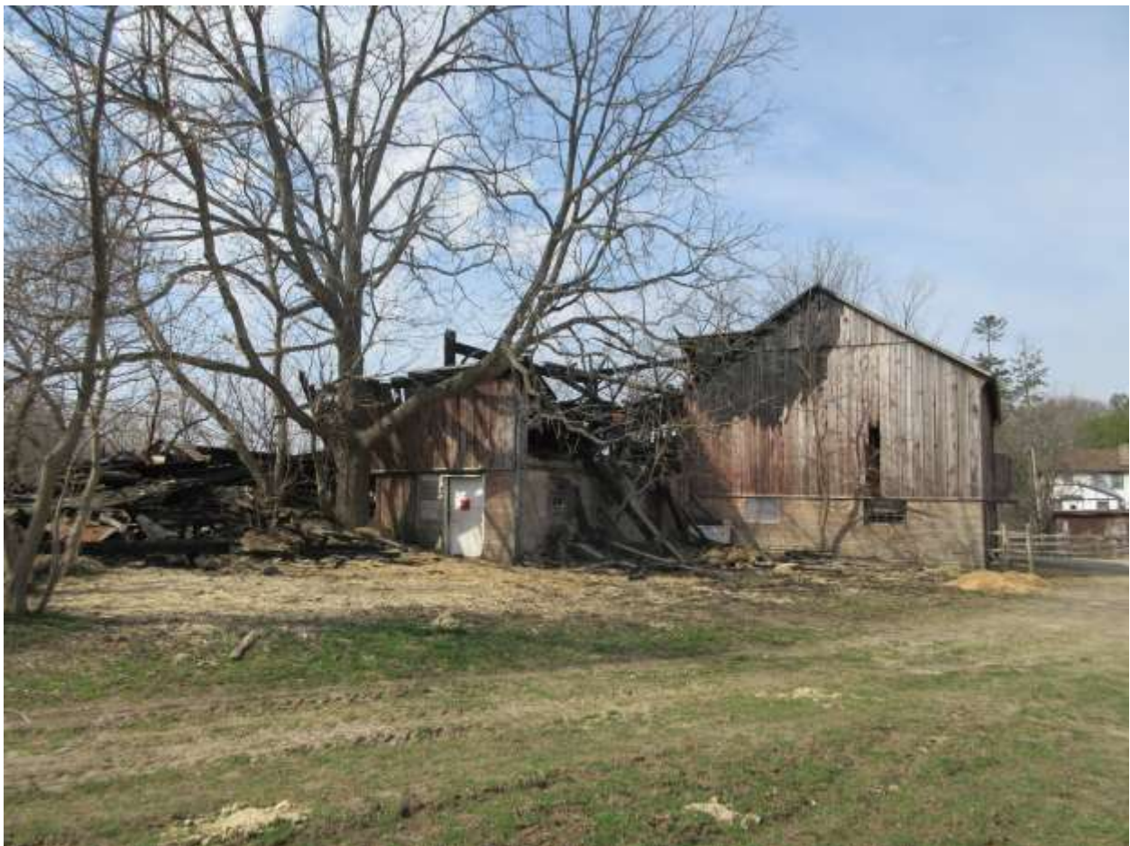
Image 12: View of the east façades of the barns located at 2154 Richmond Street. Note the extent of the damage to the south barn.
