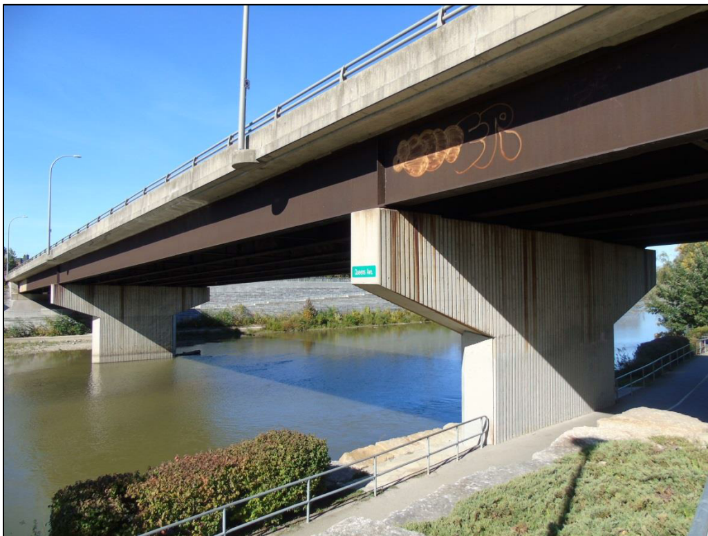
Image 11: View showing south side of The Queen's Bridge, showing piers, welded steel girders, and the TVP trail on the east side of the river
