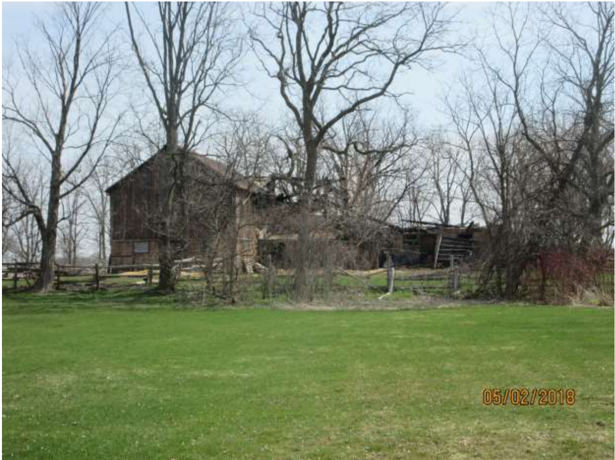
Image 11: View of the barns looking east from the south lawn of the property at 2154 Richmond Street. Note the extent of the damage to the south barn.
