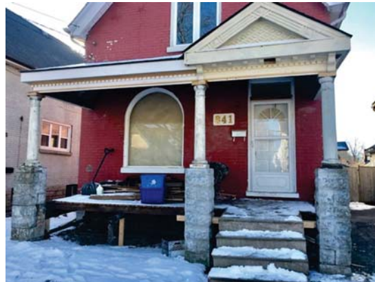
841 Princess Avenue after removal of portions of the existing porch (March 5, 2018; by applicant)
