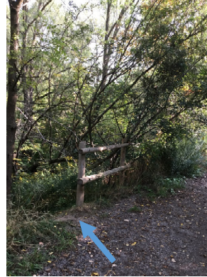
Around barrier (note lack of sign indicating closed trail)
