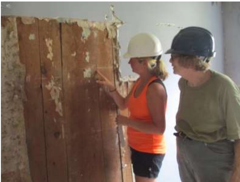
Hilary Neary and Tara Jenkins stripping wallpaper from vertical planks between two rooms in the western portion of the house
