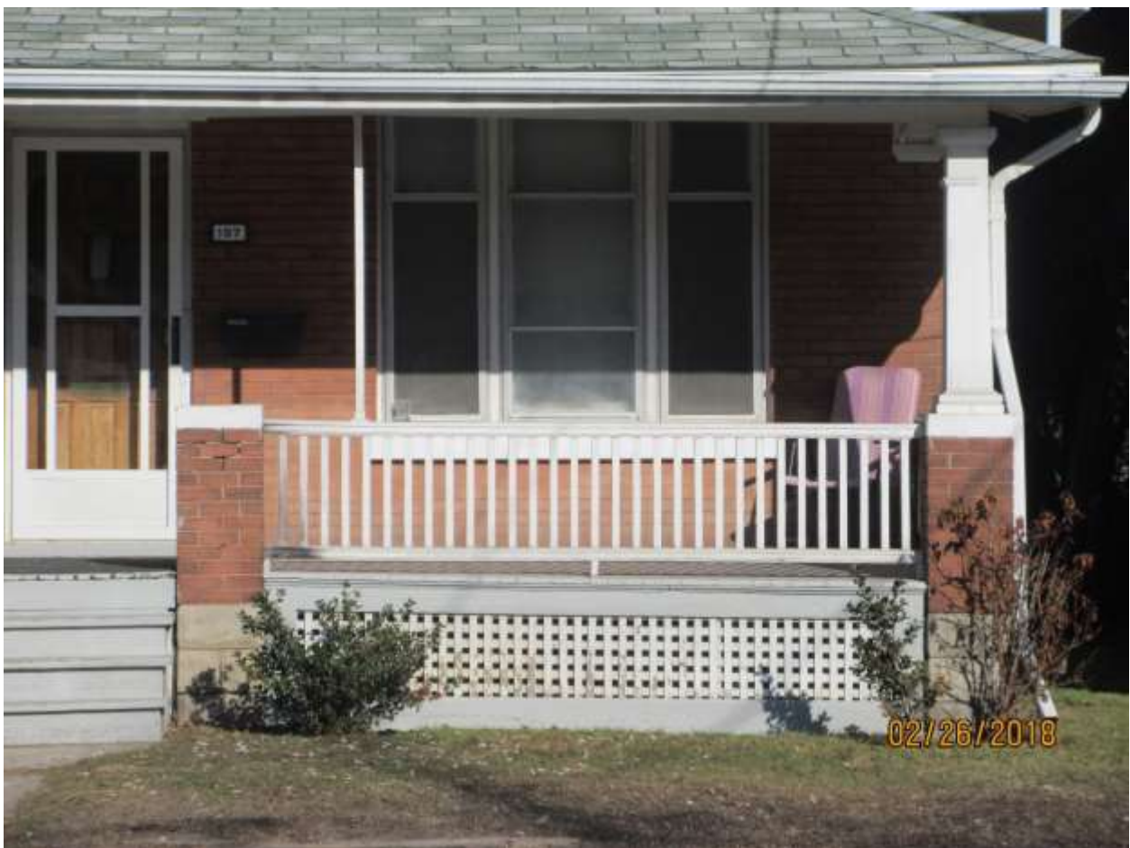
Image 8: Detail of porch balustrade at appropriate height with appropriate details and finish located at the building at 197 Wharncliffe Road North. Note the height of the balustrade is at the appropriate height to match the capstone of the brick plinths.
