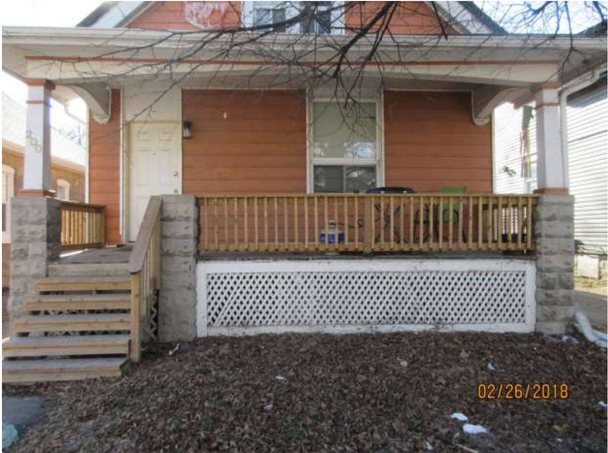
Image 5: Detail of the existing front (east) balustrade of the porch of the building at 200 Wharncliffe Road North.
