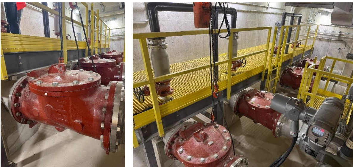
Above: Pictures of the four large pumps within the pump station that protect the underpass from flooding.
