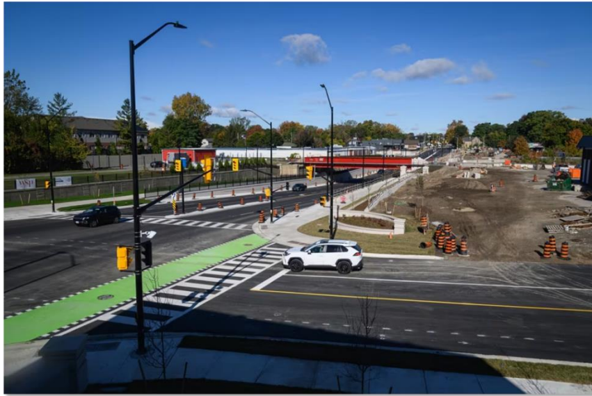
Above: Aerial view of the Adelaide Underpass open to traffic in all directions.
