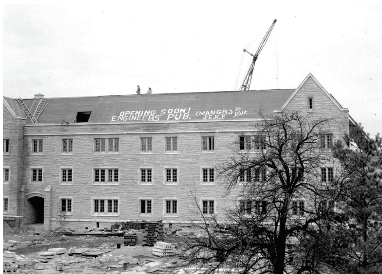
Photo 19: Photograph from 1959 of the construction of Medway Hall (Source: Free Press Collection of Negatives/ Western Archives).
