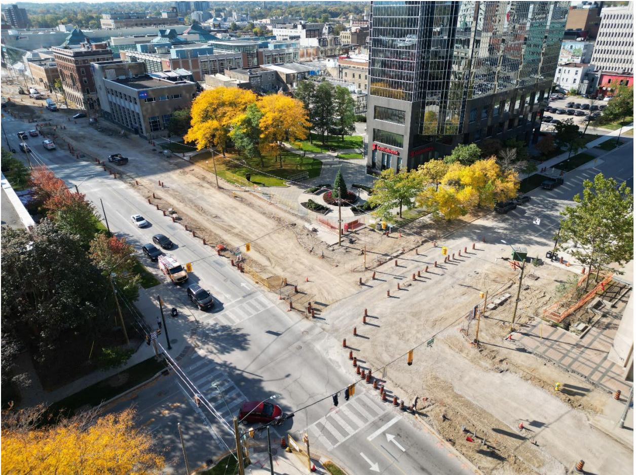
Above: Aerial view of the construction site at Wellington Street and Queens Avenue (Downtown Loop Phase 3).
