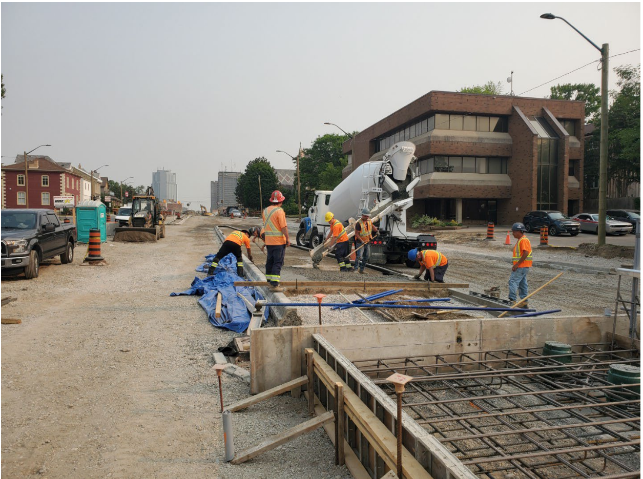
Above: Work underway to install the new bus platform at Wellington Road near South Street.
