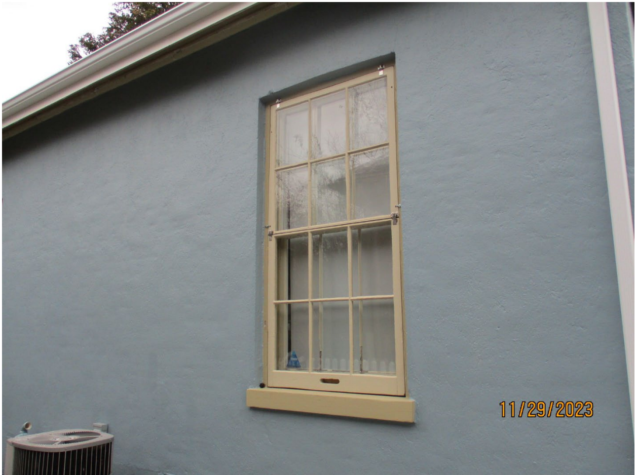
Image 35: Photograph of the six-over-six double hung painted window on east façade and wood sill on the east façade (2023).
