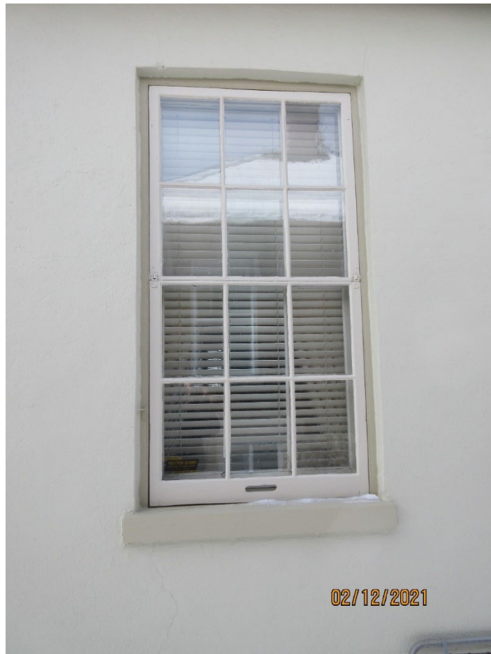
Image 34: Photograph of the six-over-six double hung painted window on east façade and wood sill on the east façade (2021).
