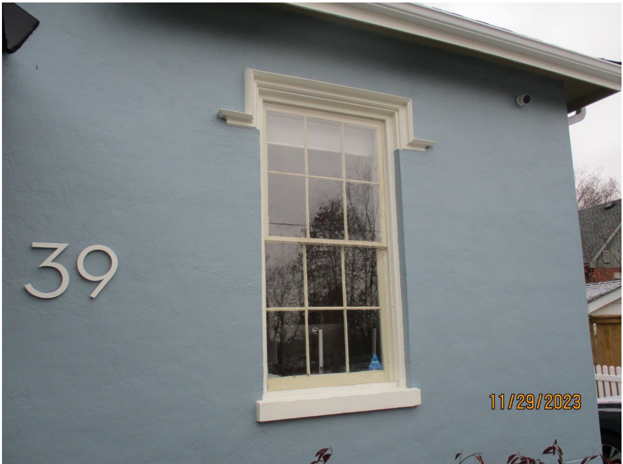
Image 24: Photograph showing the westerly front window, label, and sill of the front (north) façade of Carfrae Cottage (2023).
