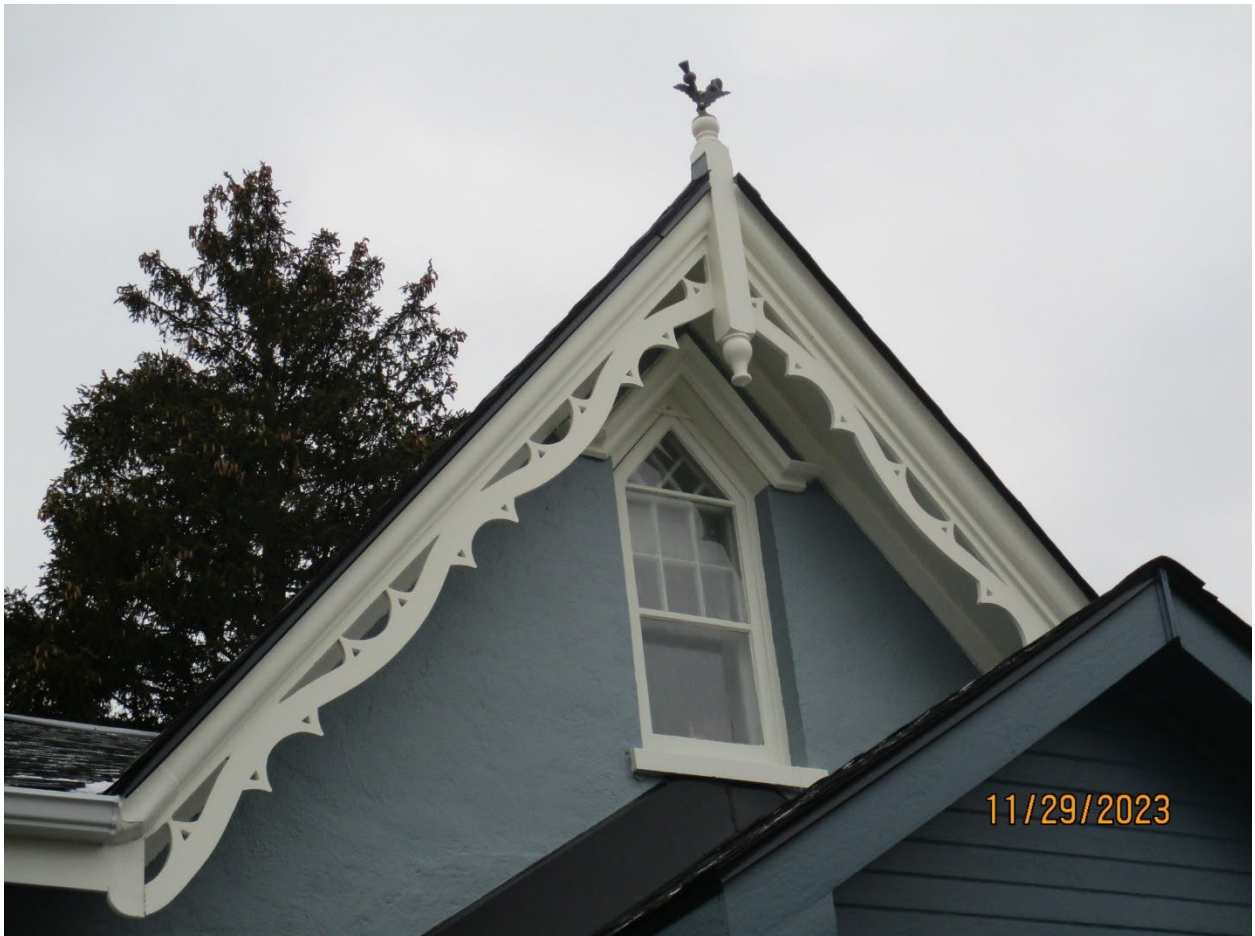
Image 26: View of the central gable dormer on the front (north) facade of Carfrae Cottage with a primitive Gothic pointed wood window. The decorative wood bargeboard of the central gable dormer is also shown, as well as the Scotch thistle (2023).
