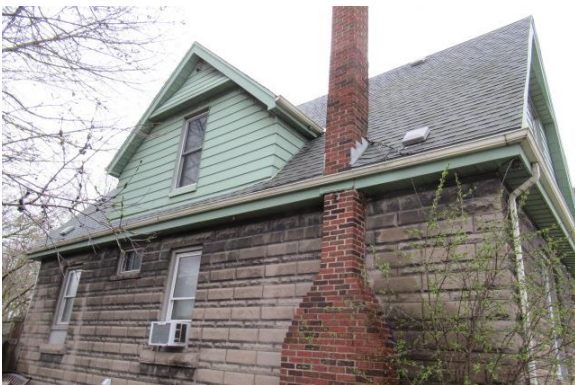
Photo Exhibit No. 3 26 Wellington – north elevation, cracking throughout brick façade.
