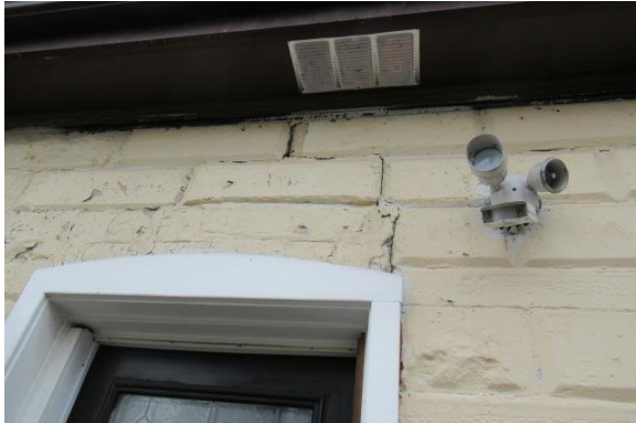
Photo Exhibit No. 7 28 Wellington – cracking through bricks at door opening.
