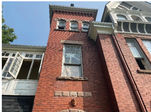
Photo 14: Middle bay of the residence on the front façade, including brick brackets, arched windows, stained-glass transom, and red stone detailing, looking north
