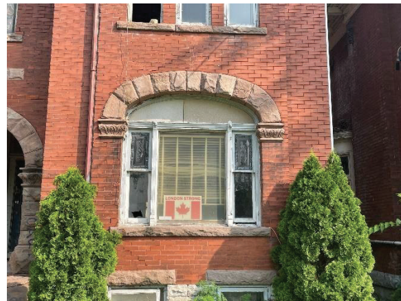
Photo 19: First storey of the eastern bay of the front façade, looking north
