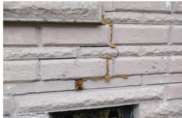
Photo Exhibit No. 18 30 Wellington – large cracks through bricks and mortar joints.
