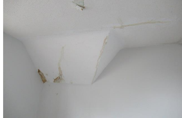
Photo Exhibit No. 22 30 Wellington – large cracks in the ceiling, along with water damage from the roof.
