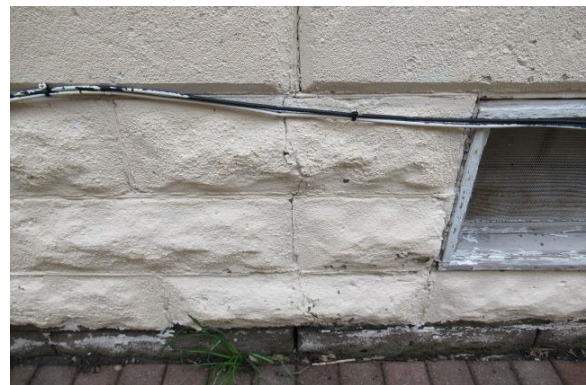
Photo Exhibit No. 6 28 Wellington – cracking through bricks.
