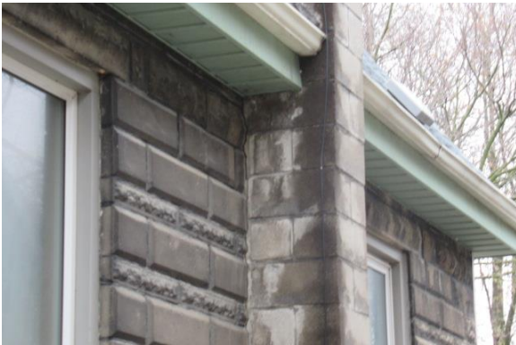
Photo Exhibit No. 2 26 Wellington – chimney is separating from main structure.
