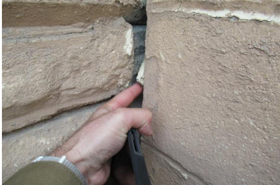
Photo Exhibit No. 19 30 Wellington – substantial separation of chimney from the structure.
