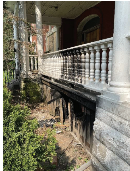
Photo 35: Evidence of fire at porch
