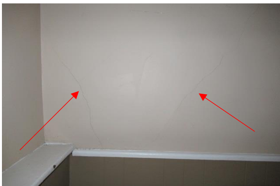
Photo Exhibit No. 9 28 Wellington – large cracks extending full wall height in stairwell walls.
