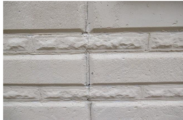
Photo Exhibit No. 5 28 Wellington – cracking through bricks.
