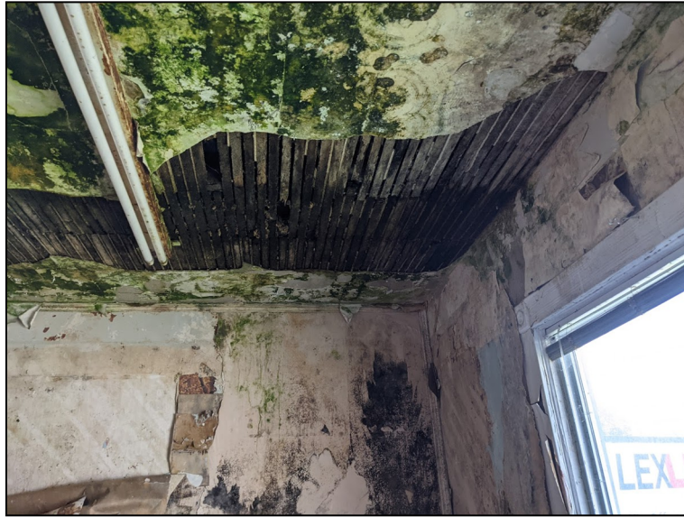
Photograph 3 – Damaged Upper Floor Framing
