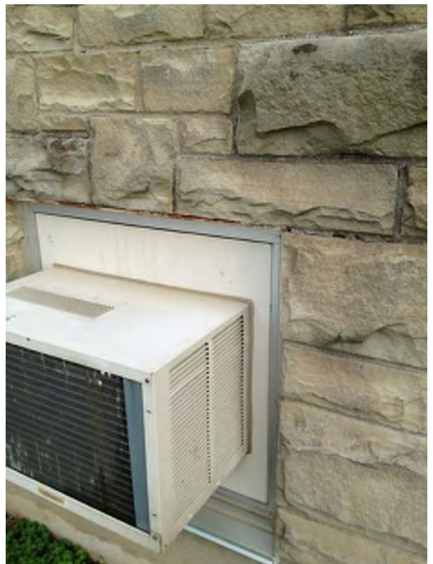
Deteriorated mortar joints on rusting steel lintel at West Elevation.
