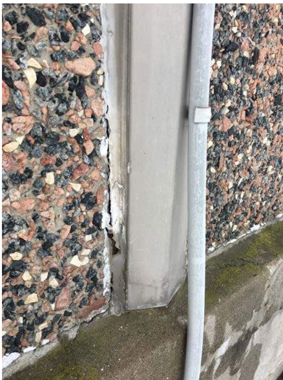
Failed caulking between precast insulated masonry panels and aluminium cover plate, east elevation of north Y-shaped wing (ERA, 2018).
