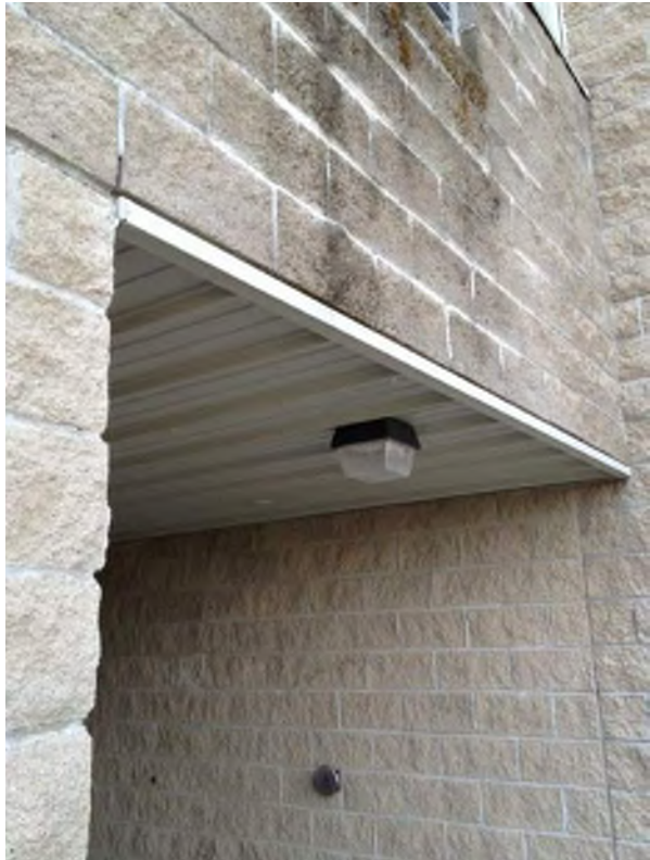
Moss growing on concrete block - 1988 addition
