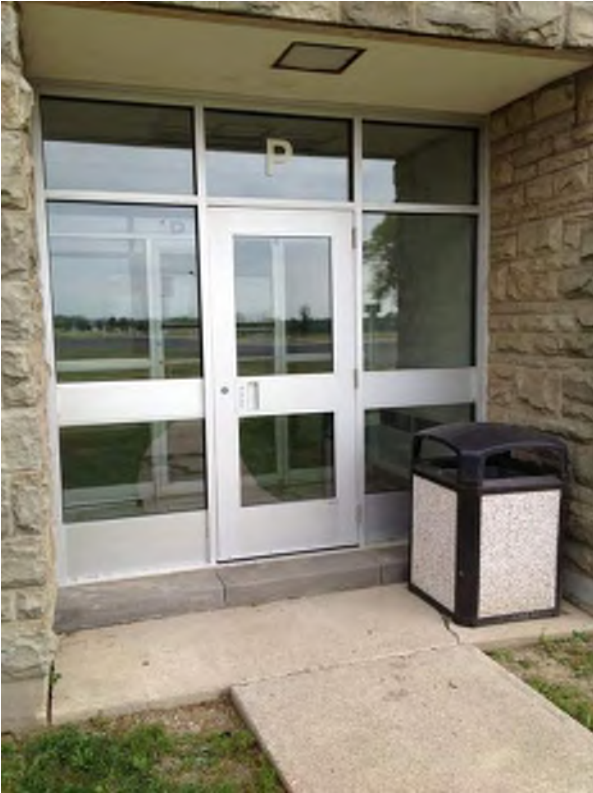
Exit P at southwest corner of technology wing does not meet current building code and does not provide barrier-free access
