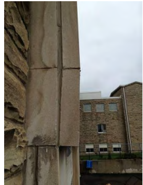
Loose smooth stone panels above Tech Wing exit and deteriorated mortar joints.
