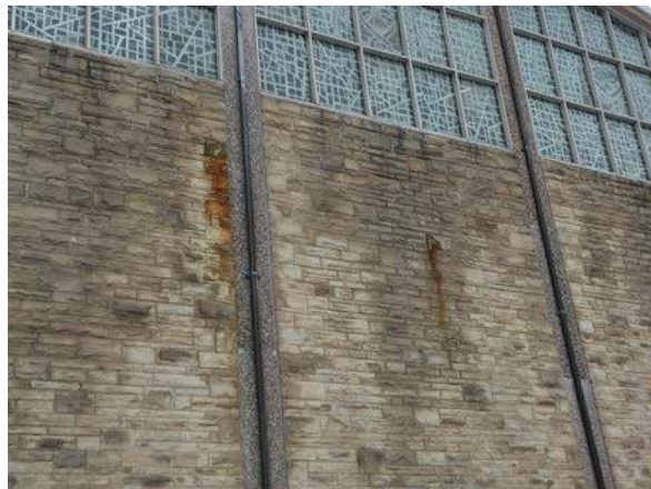
Staining and mortar loss on north chapel elevation (ERA, 2018).
