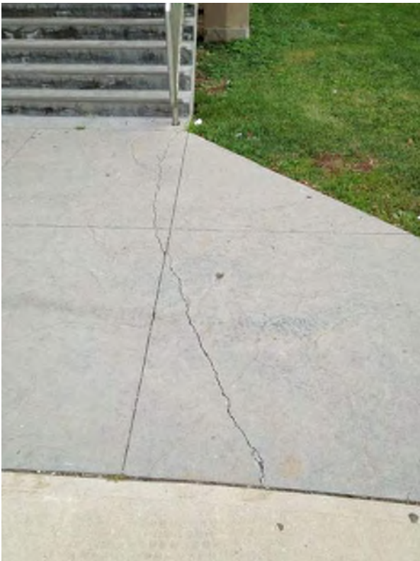
Cracked sidewalk at front entry exterior stairs
