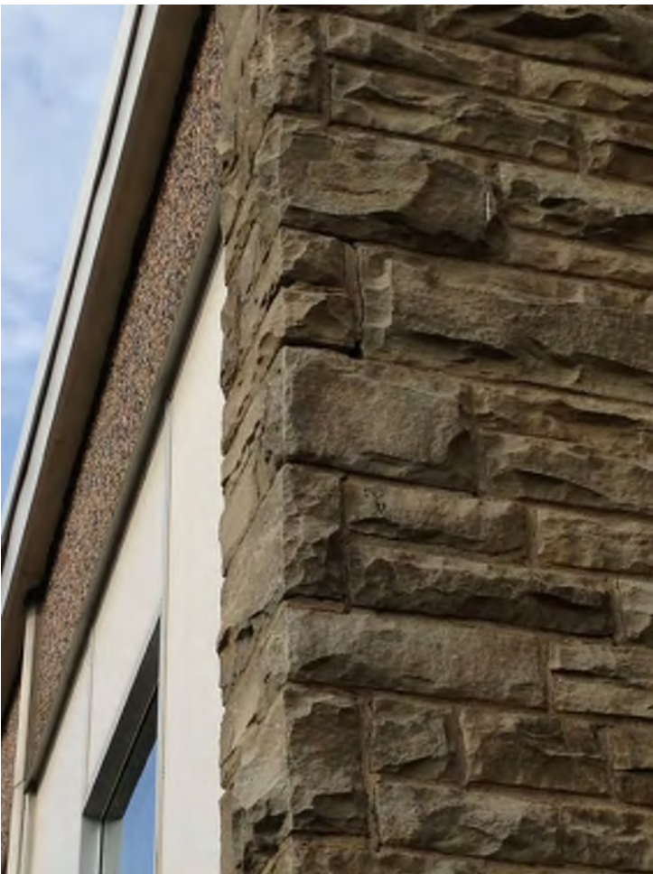
Deteriorated mortar joints and loose stones at West Elevation.
