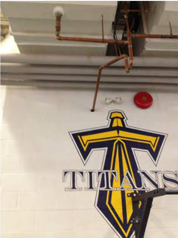
Firestopping missing at pipe penetration.
