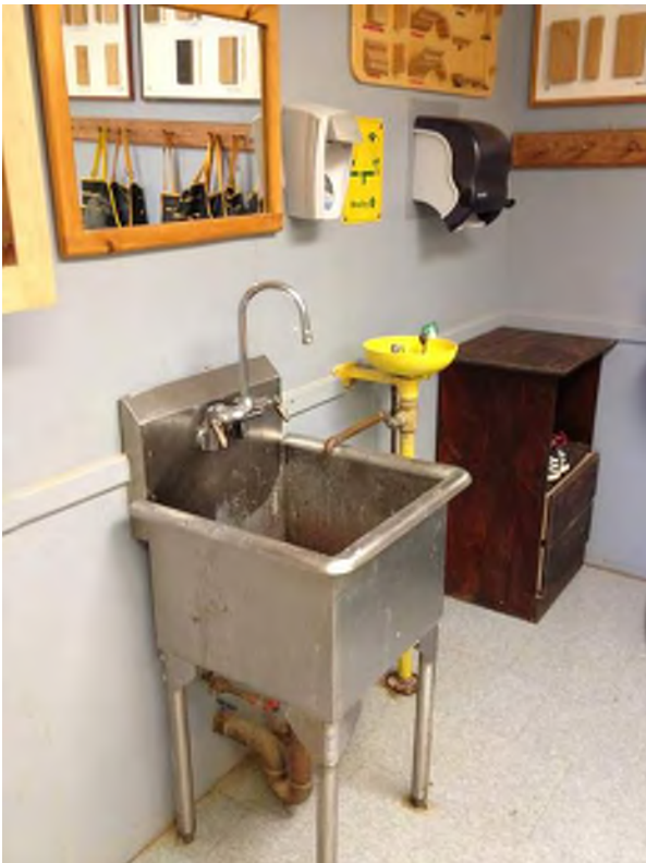
Construction Technology Classroom handwash sink.
