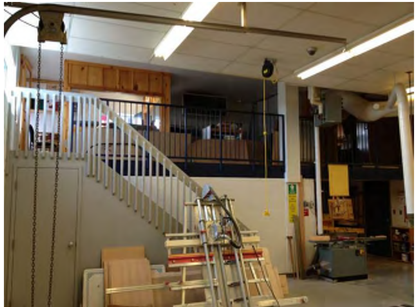
Construction Technology Classroom upper Mezzanine - Stairs are non-compliant because they are wood (combustible) construction.
