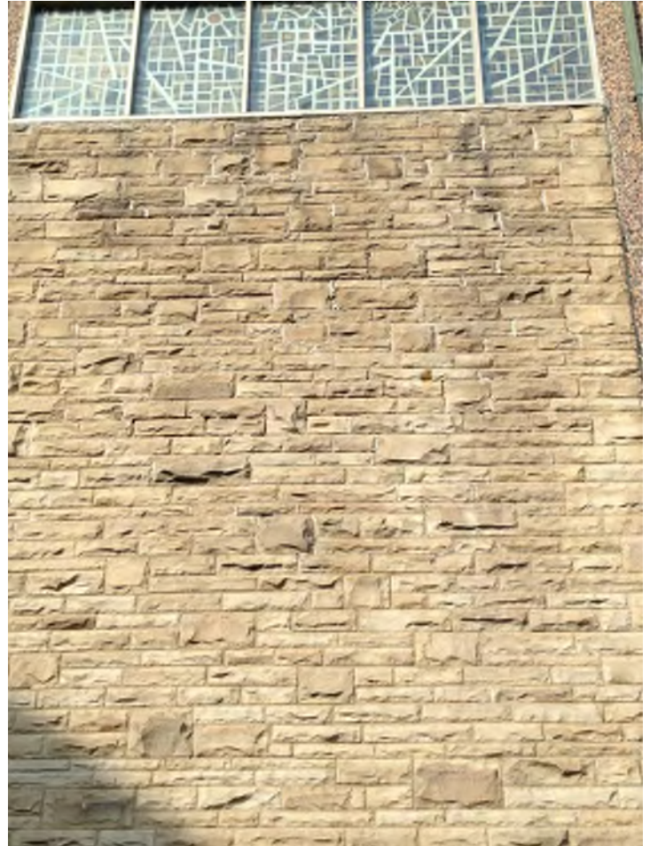
Deteriorated mortar joints on South wall of Chapel.
