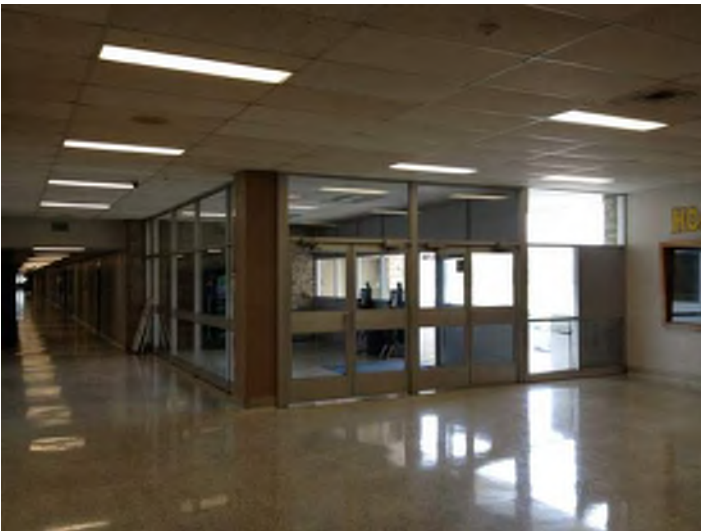
Fire exit sign missing from rear exit
