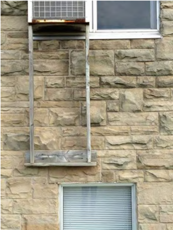
Deteriorated mortar joints below window sill on West Elevation.
