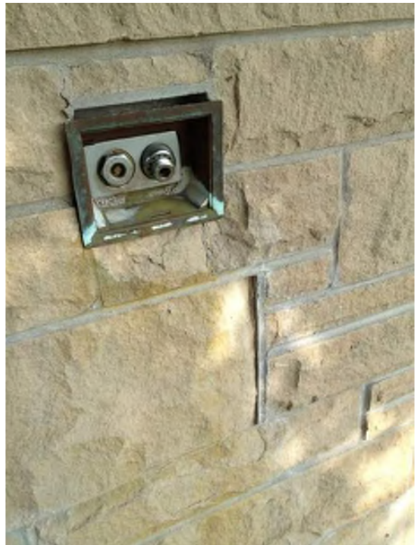
Loose hose connection box at stone - 1988 addition
