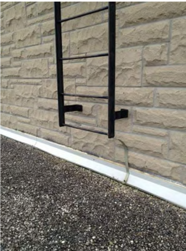
Roof Ladder at 1988 addition - height of bottom rung exceeds dimensions as per M.O.L. requirements; precast pavers over rigid insulation should be added.
