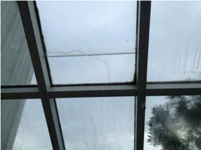
Greenhouse interior showing damaged and failed glazing units
