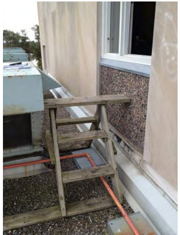
Wood platform access stair does not comply with M.O.L. requirements and is a safety hazard.
