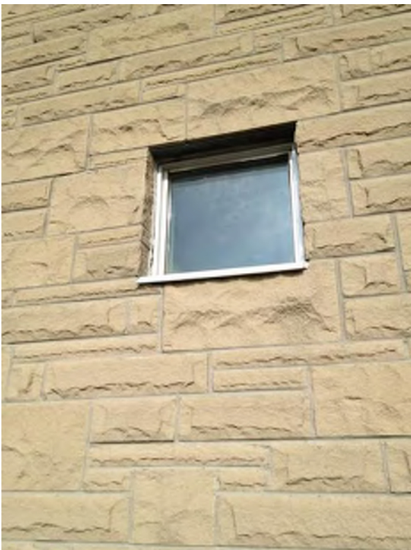
Caulked joint failure on windows on 1988 addition
