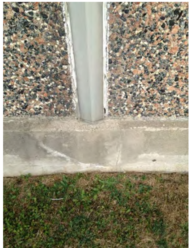
Caulked joint failure on West Elevation.
