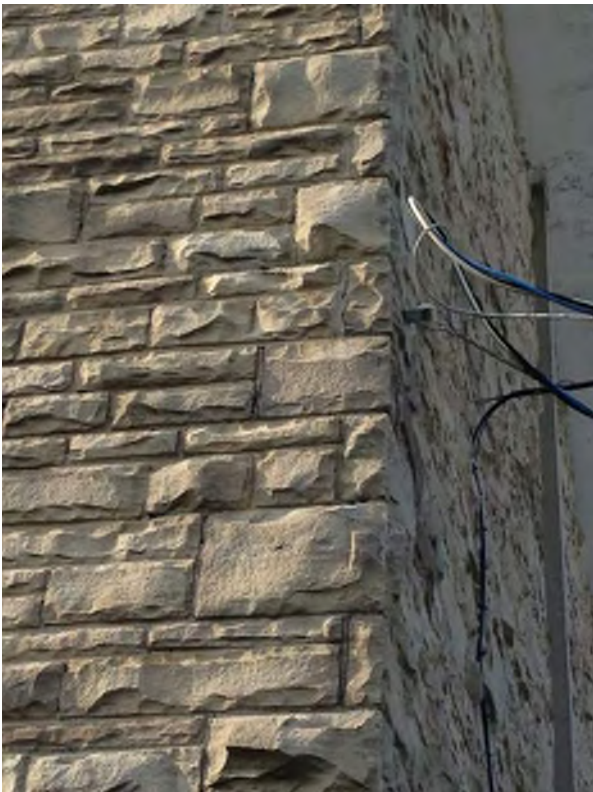
Deteriorated mortar joints - Southeast corner of Gymnasium
