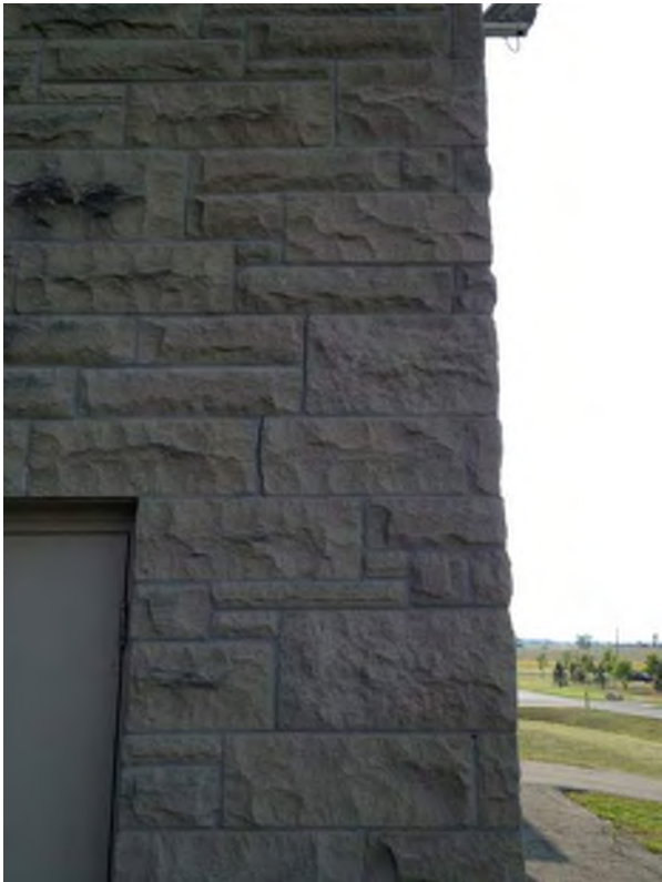
Cracked mortar joints - East Elevation - 1988 addition
