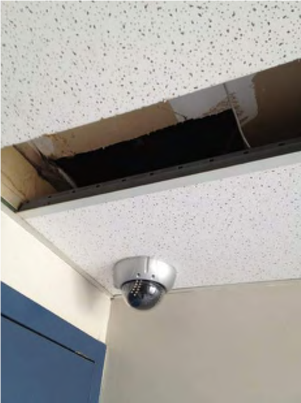
Hole in fire separation
