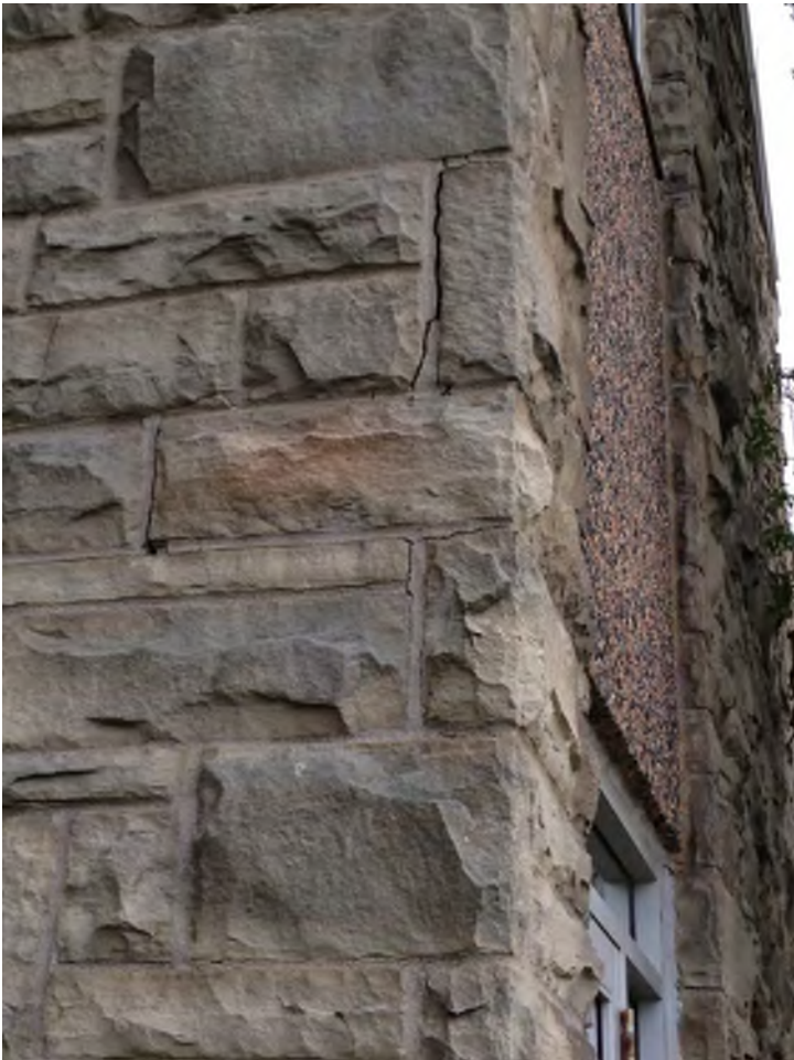
Cracked mortar joints at Tech Wing.
