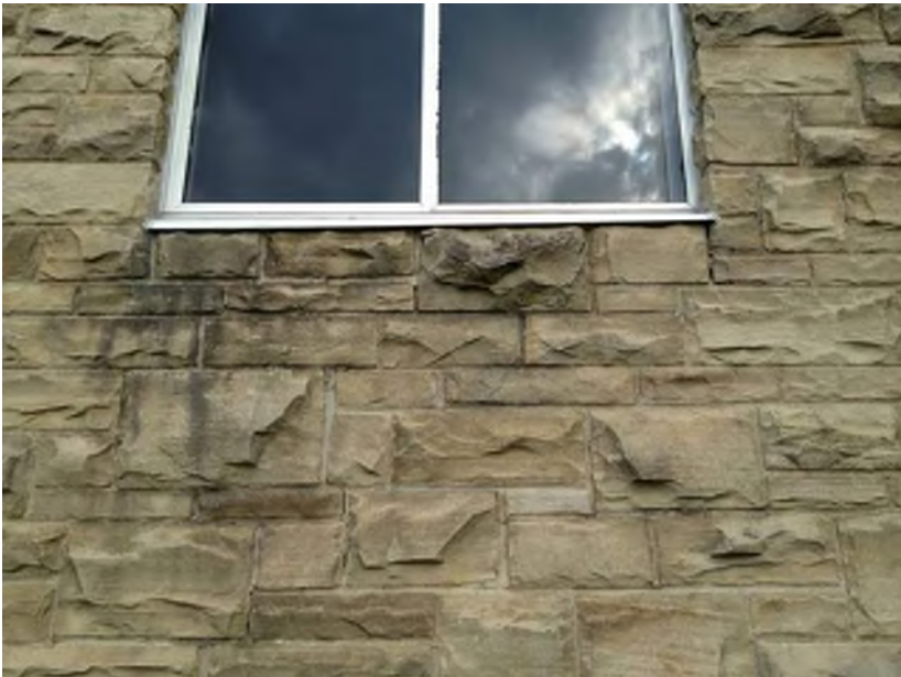
Deteriorated mortar joints below window sill on West Elevation.
