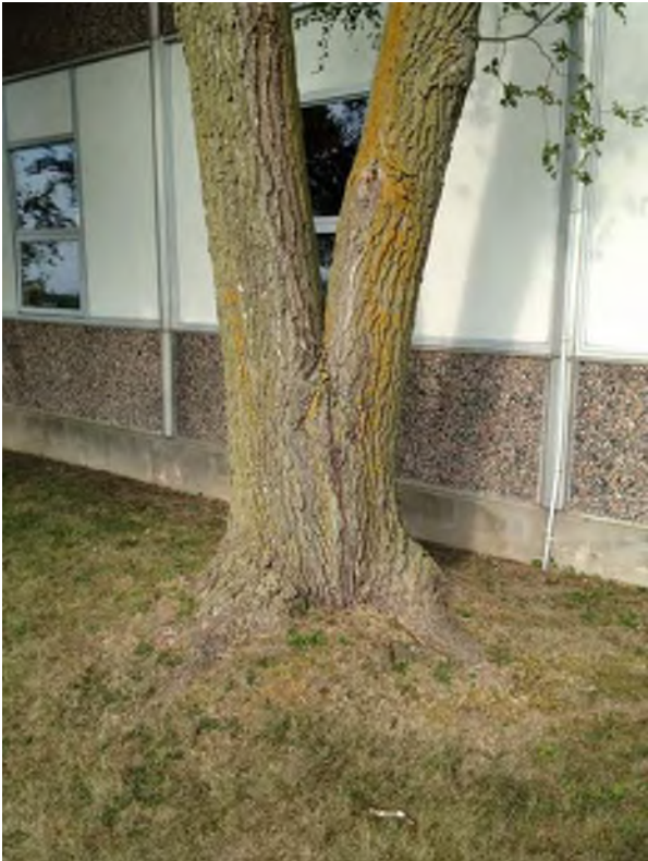
Tree in close proximity to West building wall and notch susceptible to water intrusion and rot.
