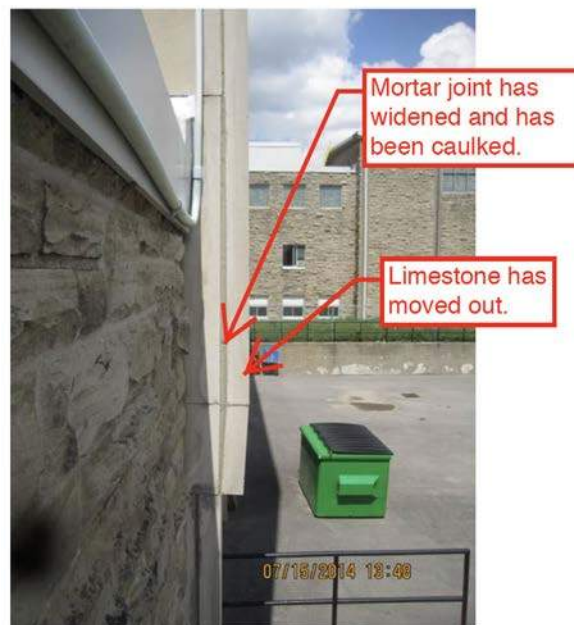
Photo of bulging limestone panel at southeast corner of three-storey block (Hastings & Aziz, 2014).
