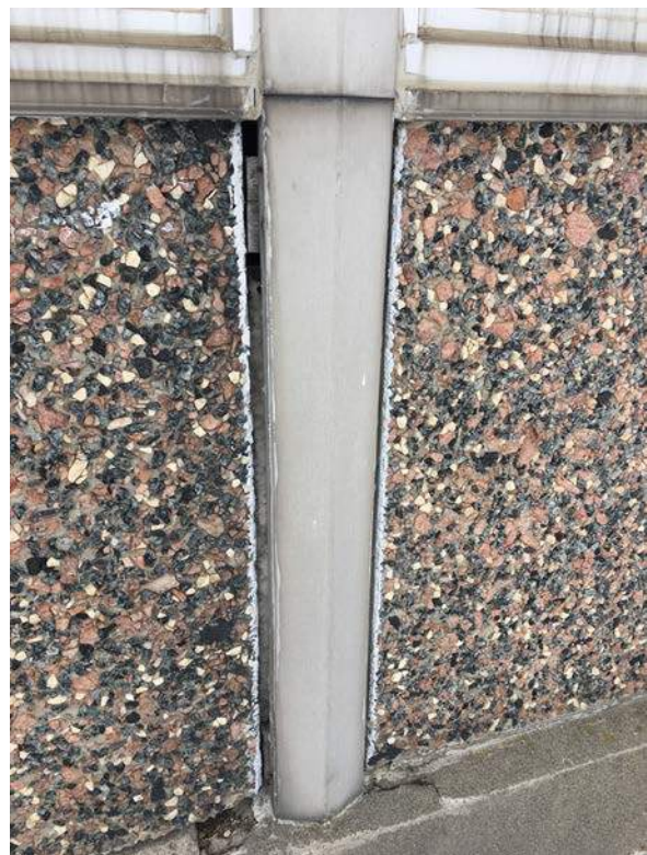
Wall cavity exposed due to gap between precast insulated masonry panels and aluminium cover plate, east elevation of north Y-shaped wing (ERA, 2018).
