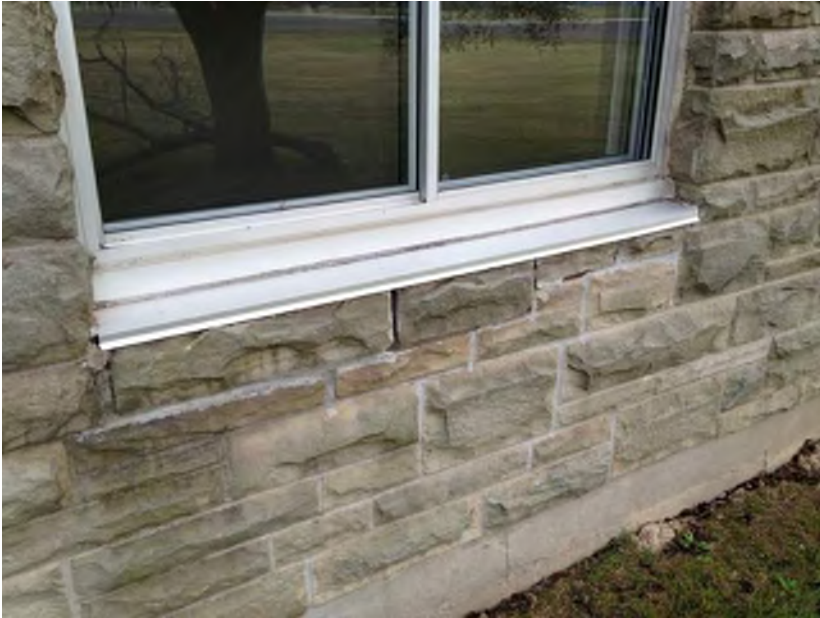
Deteriorated mortar joints below window sill in Tech Wing.
