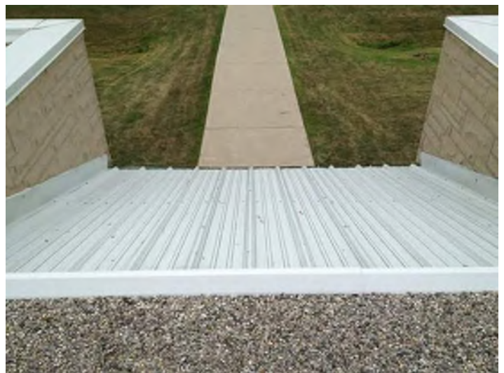
Sloped roof over exit without snow guards
