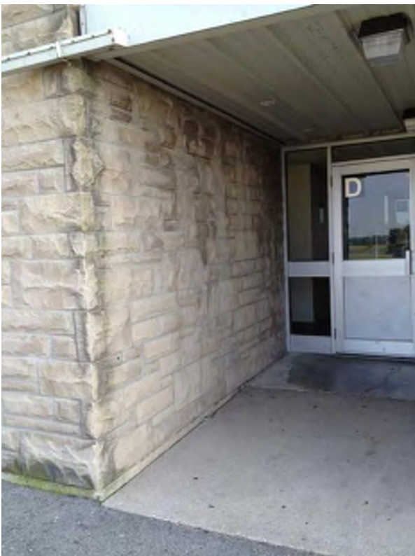
Water damage below soffit - North Elevation 1988 addition
