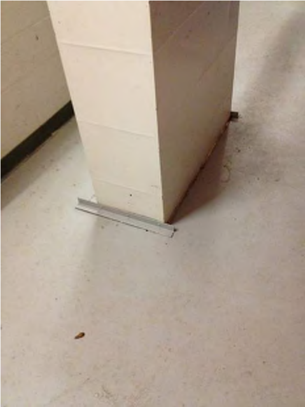
Duct penetration at fire-rated floor not firestopped; damper missing
