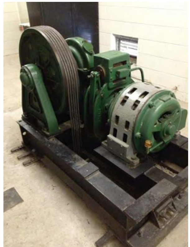
Elevator Machine Room Equipment
