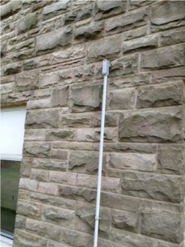
Caulking joint missing at conduit penetration
