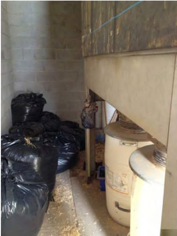
Dust collector interior
