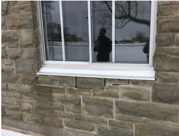
Mortar loss below window on original south Y-shaped block, west elevation (ERA, 2018).
