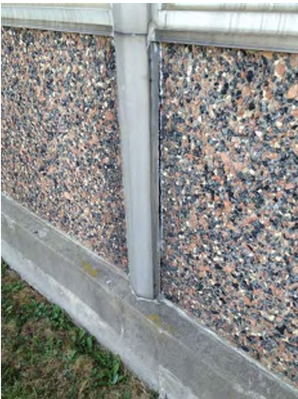
Caulked joint failure on East Elevation
