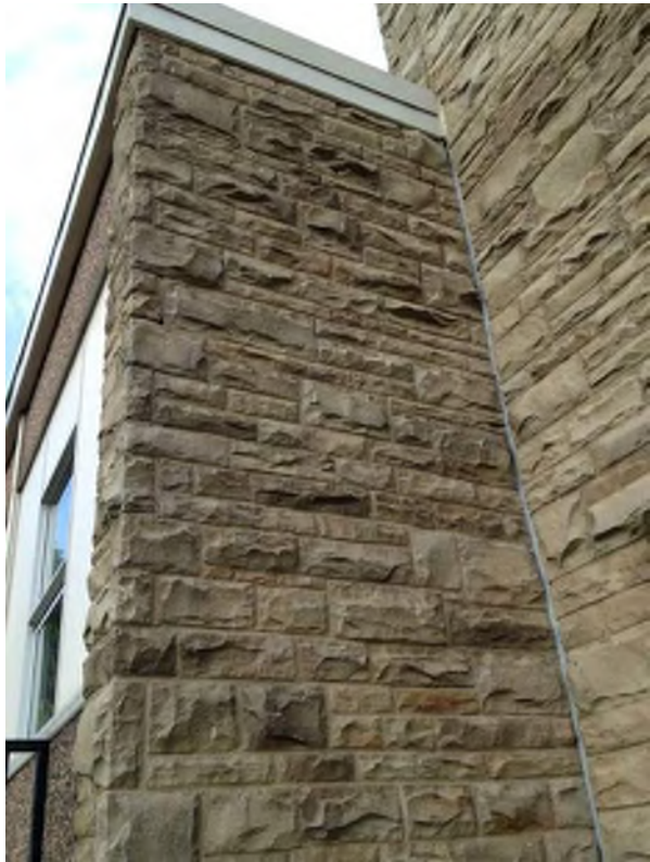
Deteriorated mortar joints on West Elevation.
