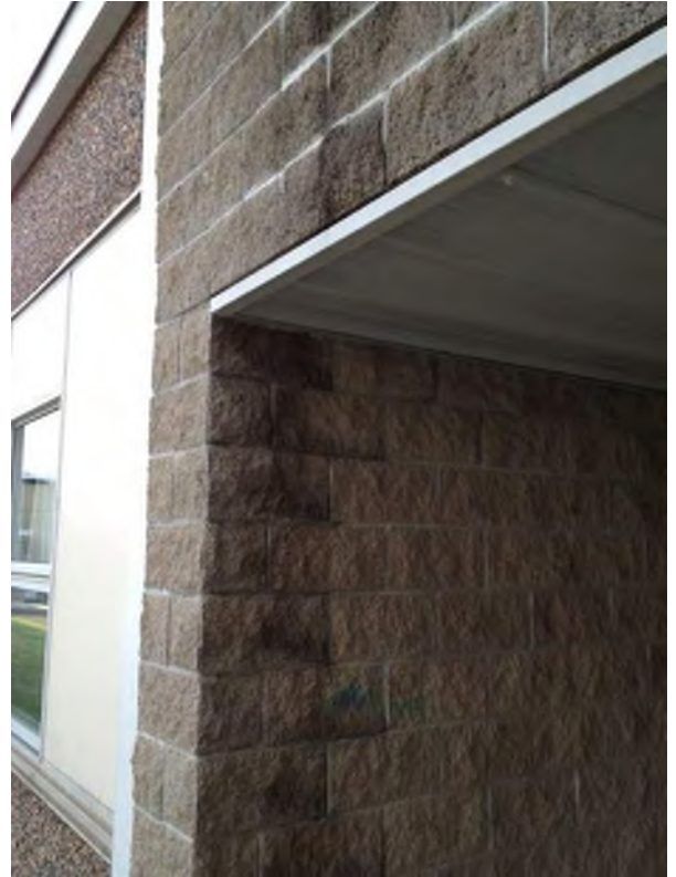
Water damage at soffit - East Elevation 1988 addition
