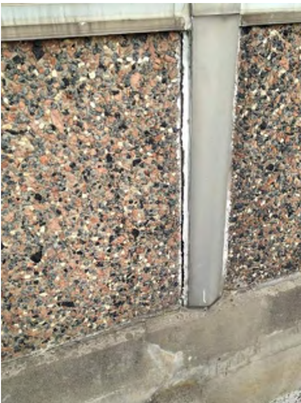
Caulked joint failure on West Elevation.
