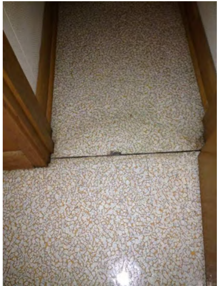
Existing asbestos containing flooring in chapel.
