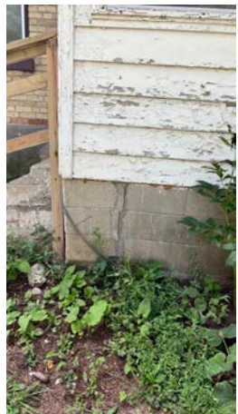
85. 7056 Pack Rd Cracked Cinder Block Mudroom Foundation.HEIC
