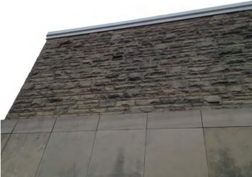
Exterior stone at Elevator Machine Room - weathered and showing signs of cracking to mortar joints.
