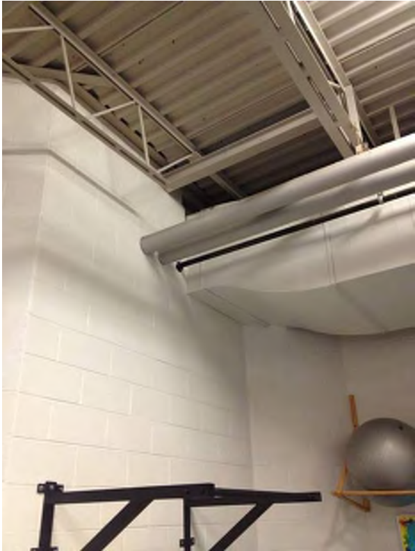
Firestopping missing and fire separation incomplete.
