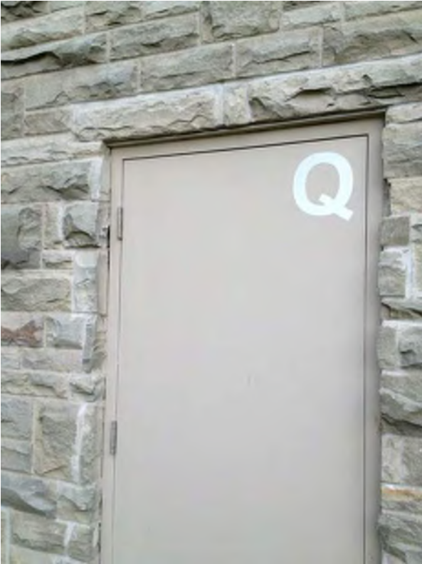
Exit door missing caulking in Tech Wing - large gap allows moisture at penetration.
