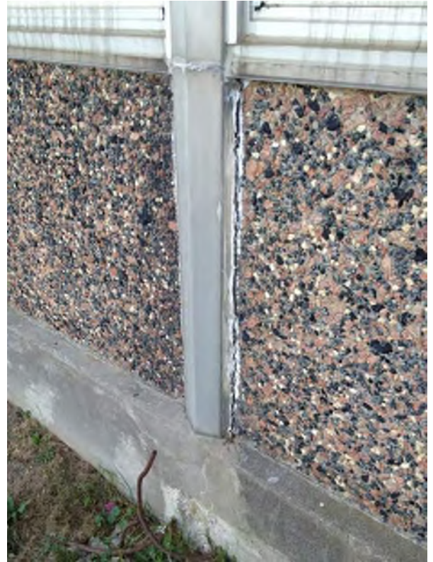
Caulked joint failure on East Elevation. Note projecting steel bars below present safety hazard.
