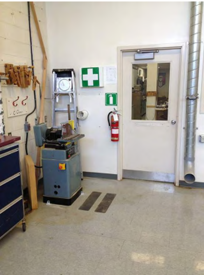
Fabrication Room - equipment located too close to egress door from adjacent teaching space.
