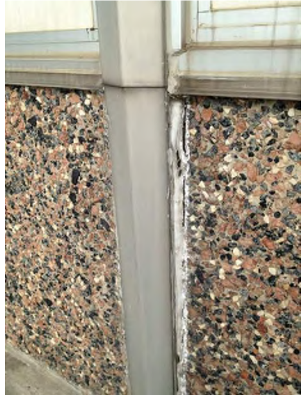
Caulked joint failure on West Elevation
