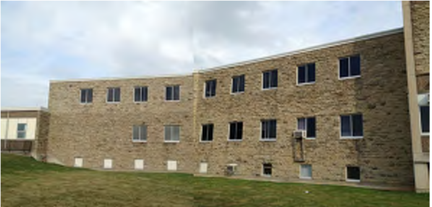
Partial West Elevation - area of deteriorated mortar joints below all window sills.
