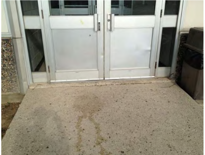
Entrance door from barrier-free parking spaces - concrete sidewalk had settled - does not meet current building code
