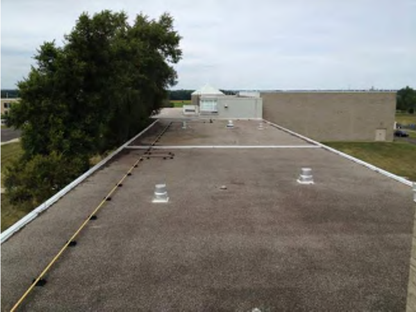
Overhanging trees at Roof H
