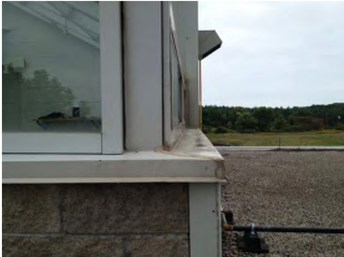
Greenhouse sill provides inadequate slope to shed water onto roof below.
