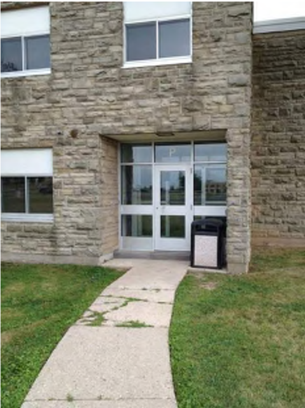
Damaged Sidewalk at Tech Wing Exit
