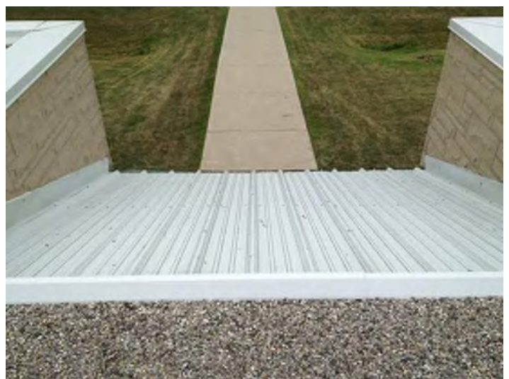
Sloped roof over exit without snow guards
