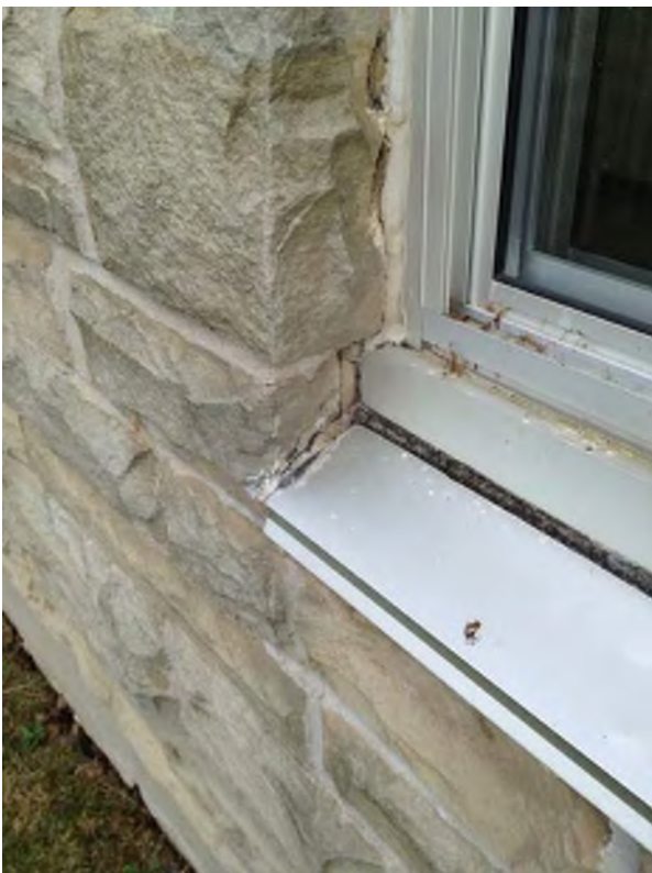
Window jamb and sill caulking - Tech Wing - sills should have end dams.
