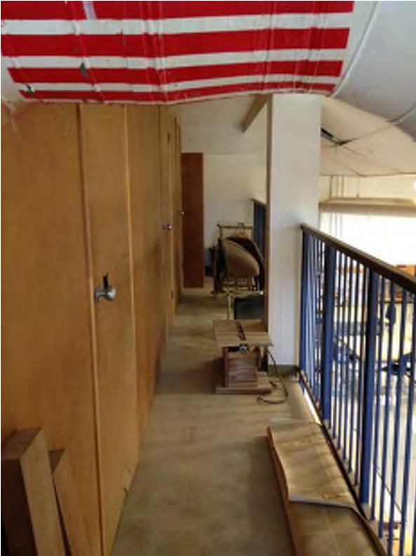
Construction Technology Classroom upper Mezzanine with low head clearance at ductwork
