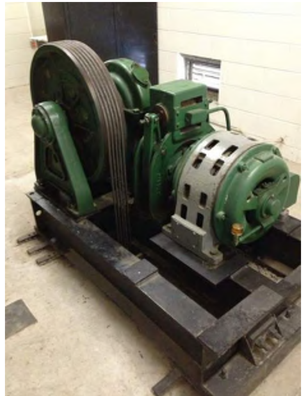
Elevator Machine Room Equipment
