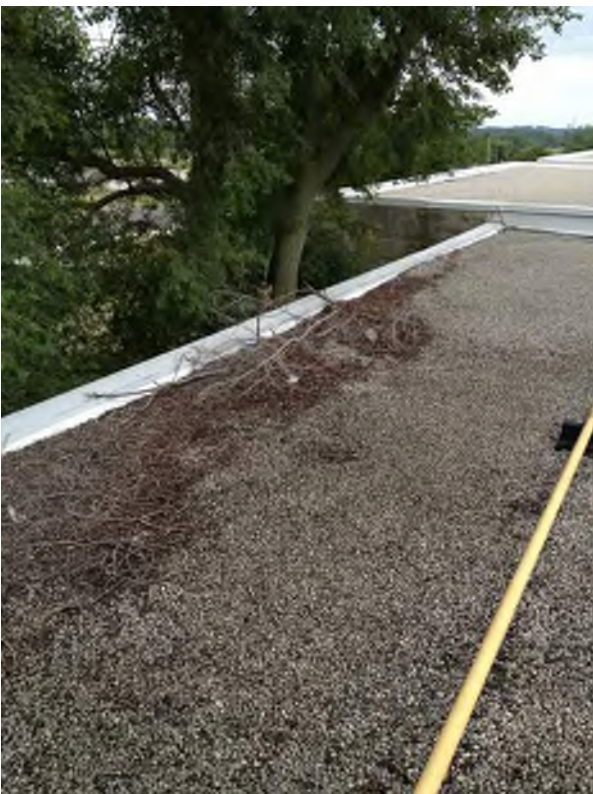
Debris at overhanging trees on Roof H
