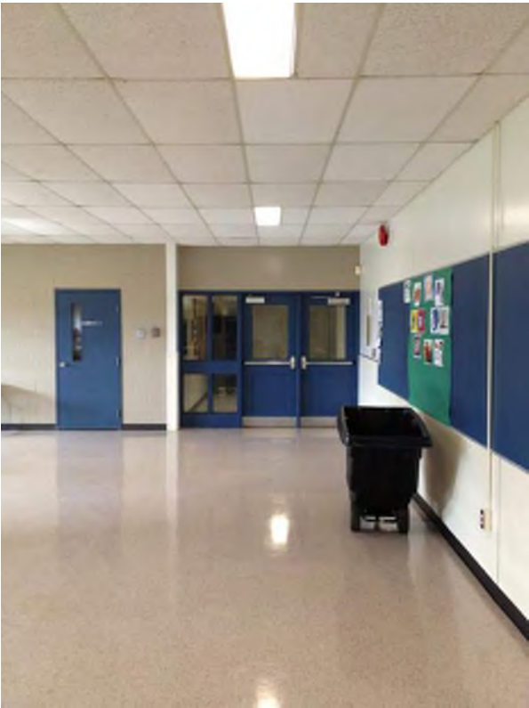
Fire exit sign missing in cafeteria
