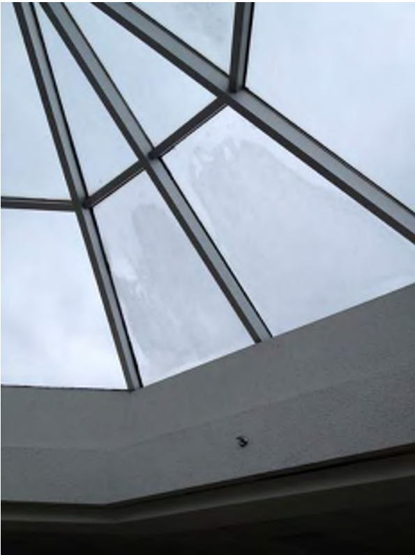
Library skylight interior showing failed glass units.
