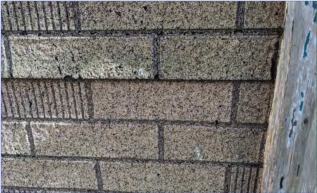
Photo 15: Detailed view of the insulbrick type cladding on the enclosed front porch area on the south elevation
