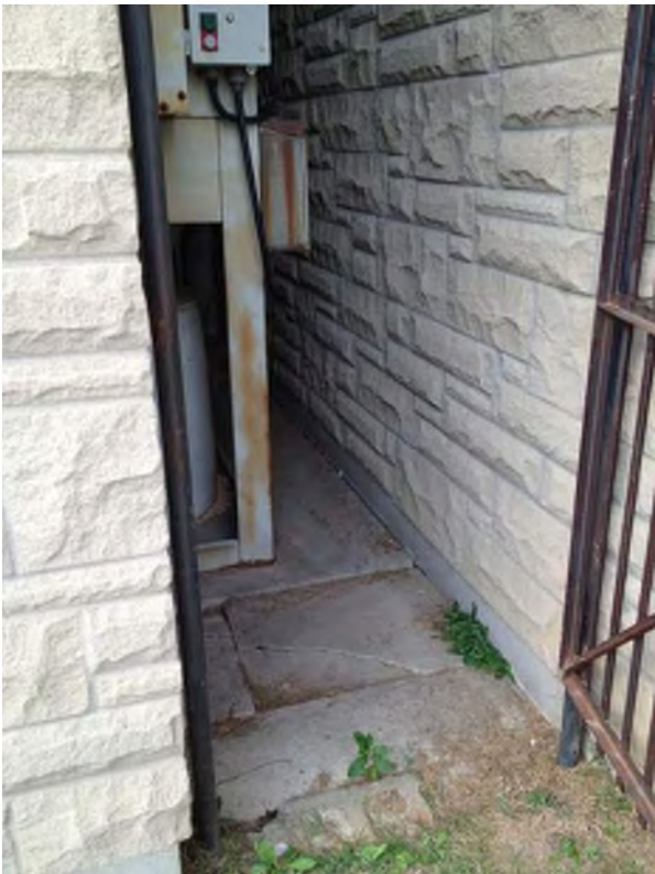
Dust collector enclosure access.
