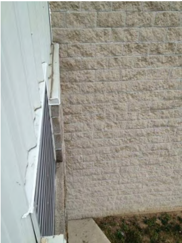
Metal flashing and sill missing from bottom of louvre
