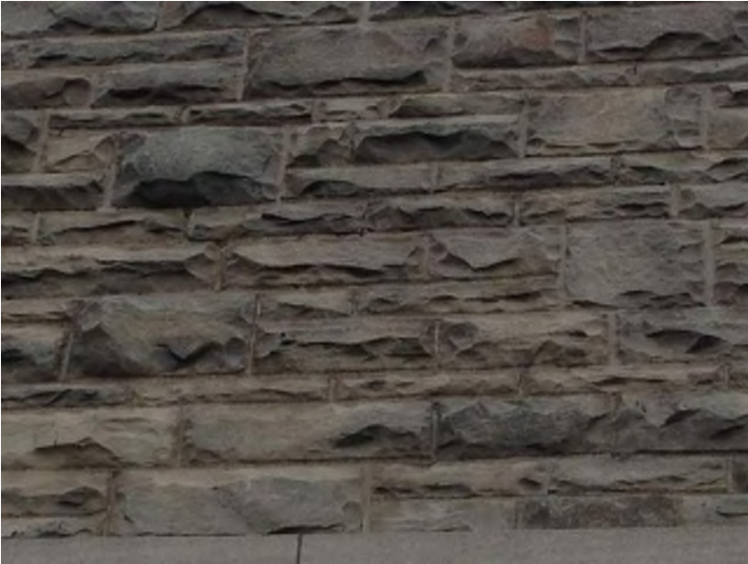
Exterior stone at Elevator Machine Room - mortar joints beginning to crack and deteriorate.
