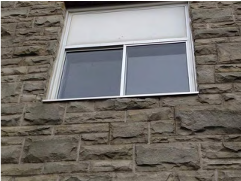
Loose mortar joints below window sill on second floor Tech Wing from water penetration.
