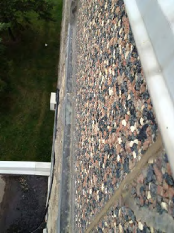
Exterior metal sill at precast panel - joints have failed and does not project past stone below causing staining and water to deteriorate mortar joints
