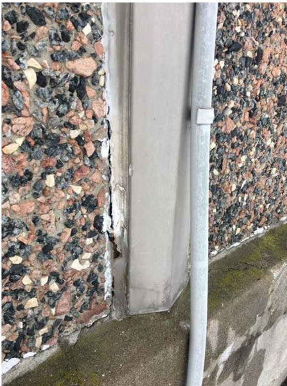
Failed caulking between precast insulated masonry panels and aluminium cover plate, east elevation of north Y-shaped wing (ERA, 2018).
