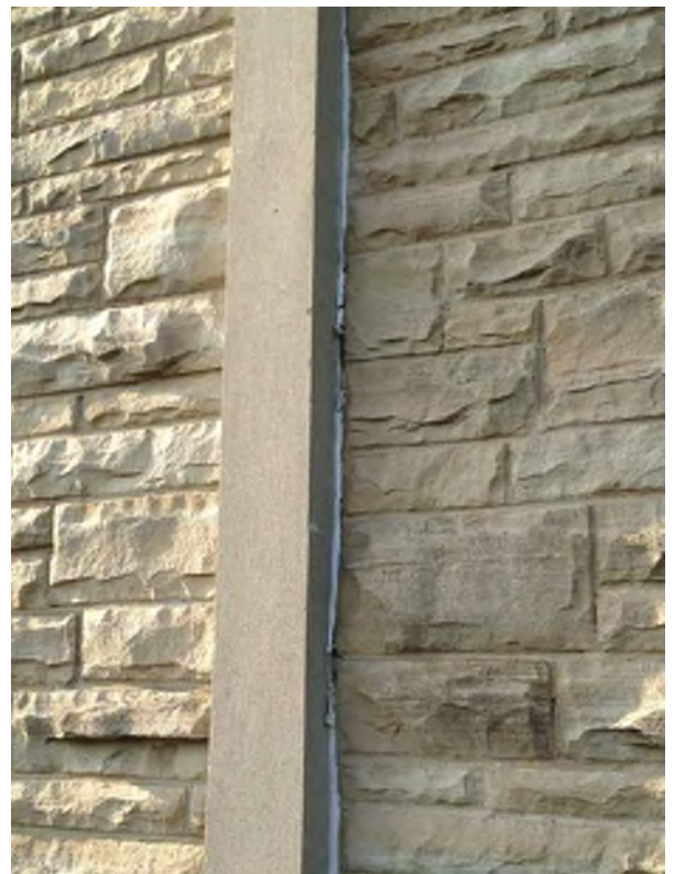
Caulking joint at Gymnasium Wall - South Elevation
