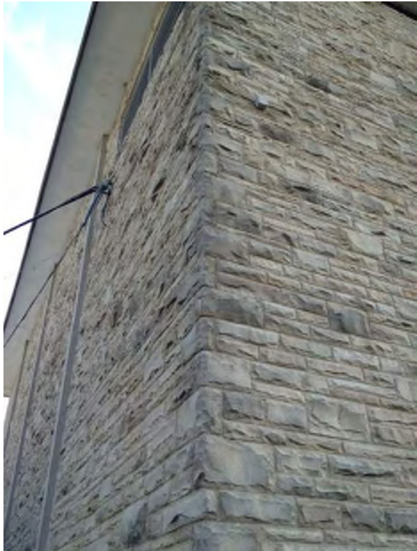
Cracked mortar joints - Gymnasium East elevation
