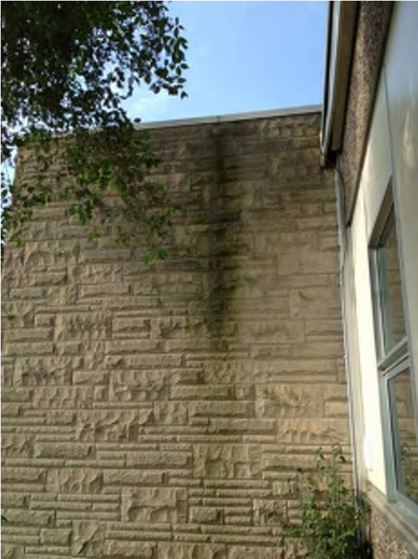
Staining on stone from metal flashing joint above - 1988 addition
