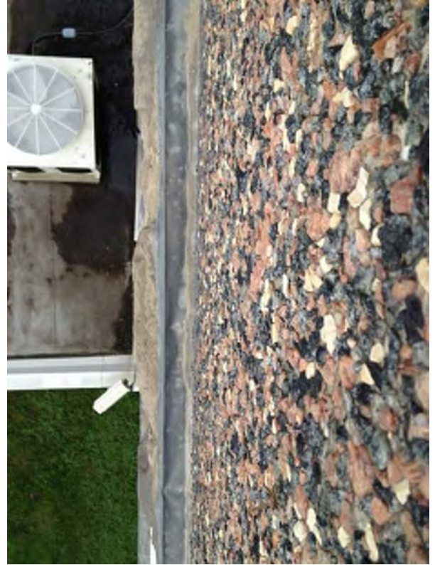
Exterior metal sill at precast panel - joints have failed and does not project past stone below causing staining and water to deteriorate mortar joints
