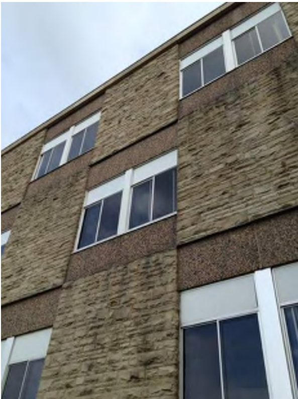
Horizontal sills at panels do not project past rough failed stone causing staining and weathering of stone and mortar joints.
