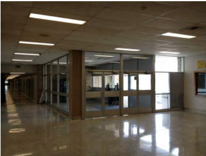
Fire exit sign missing from rear exit
