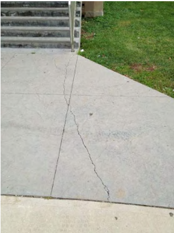
Cracked sidewalk at front entry exterior stairs
