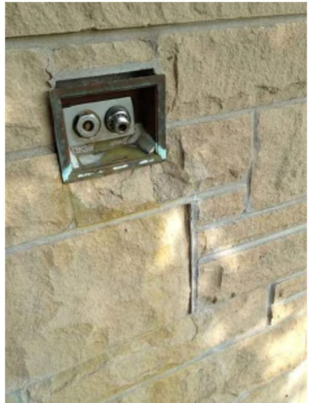
Loose hose connection box at stone - 1988 addition
