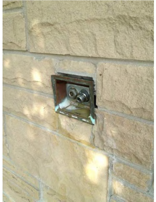
Loose hose connection box at stone - 1988 addition
