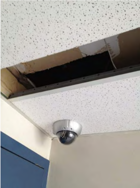
Hole in fire separation
