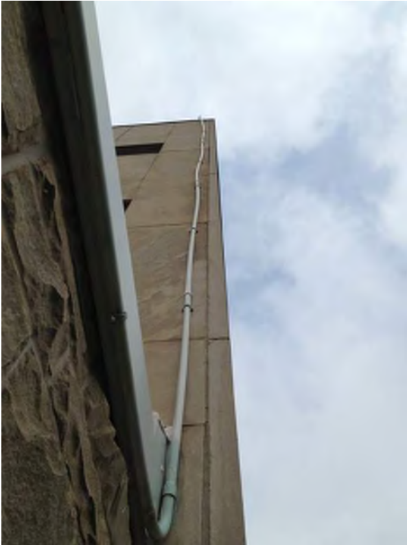
Deteriorated mortar joints at South Elevation
