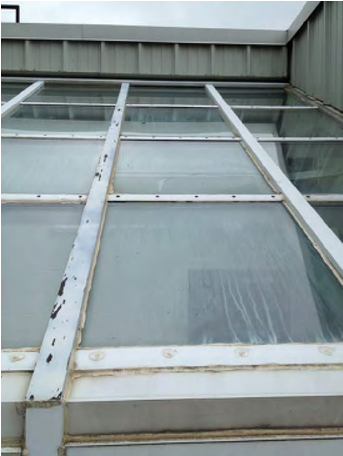
Greenhouse showing damaged and failed glazing units.
