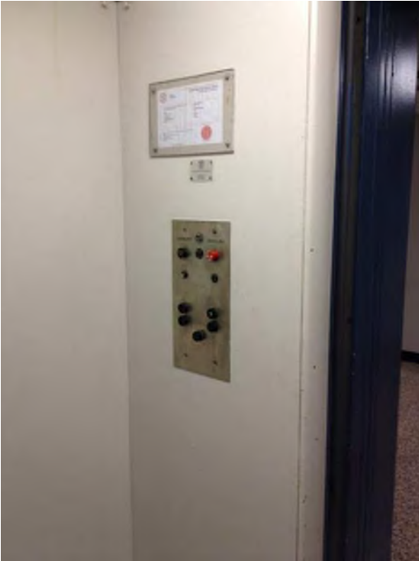
Elevator interior cab panel
