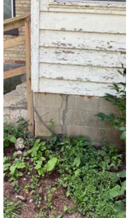
85. 7056 Pack Rd Cracked Cinder Block Mudroom Foundation.HEIC
