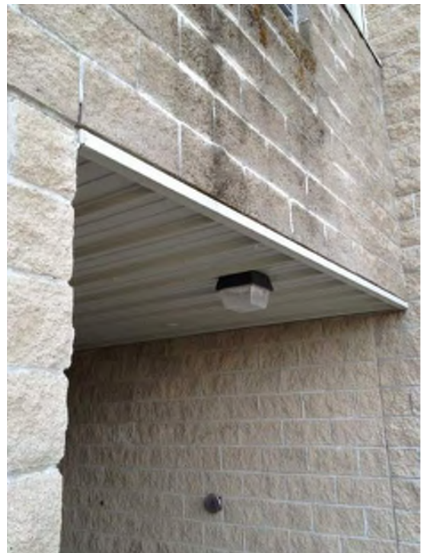
Moss growing on concrete block - 1988 addition
