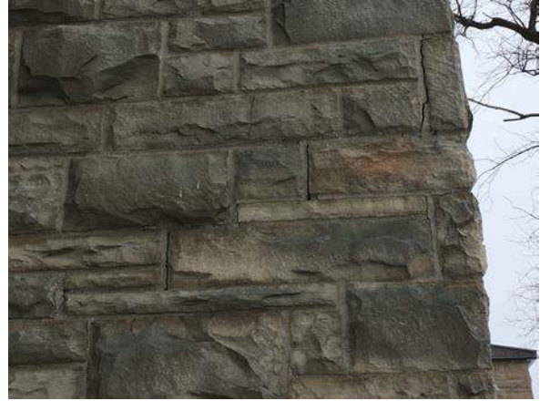
Mortar loss on wall, original south Y-shaped block, west elevation (ERA, 2018).
