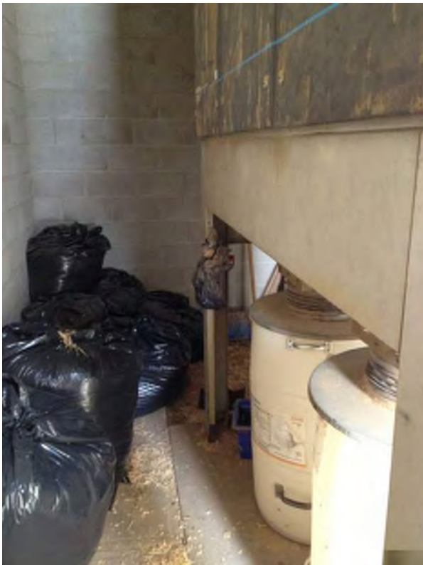
Dust collector interior
