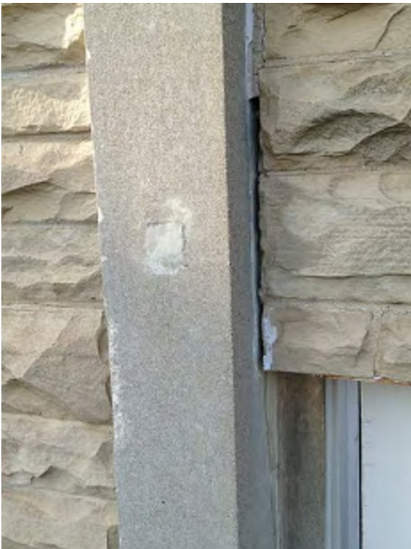
Caulked joint at Gymnasium wall window head - South Elevation. Note deterioration of mortar joints
