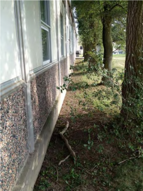
Tree at West Elevation too close to building and branches beginning to decay and fall.
