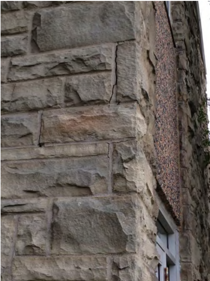
Cracked mortar joints at Tech Wing.
