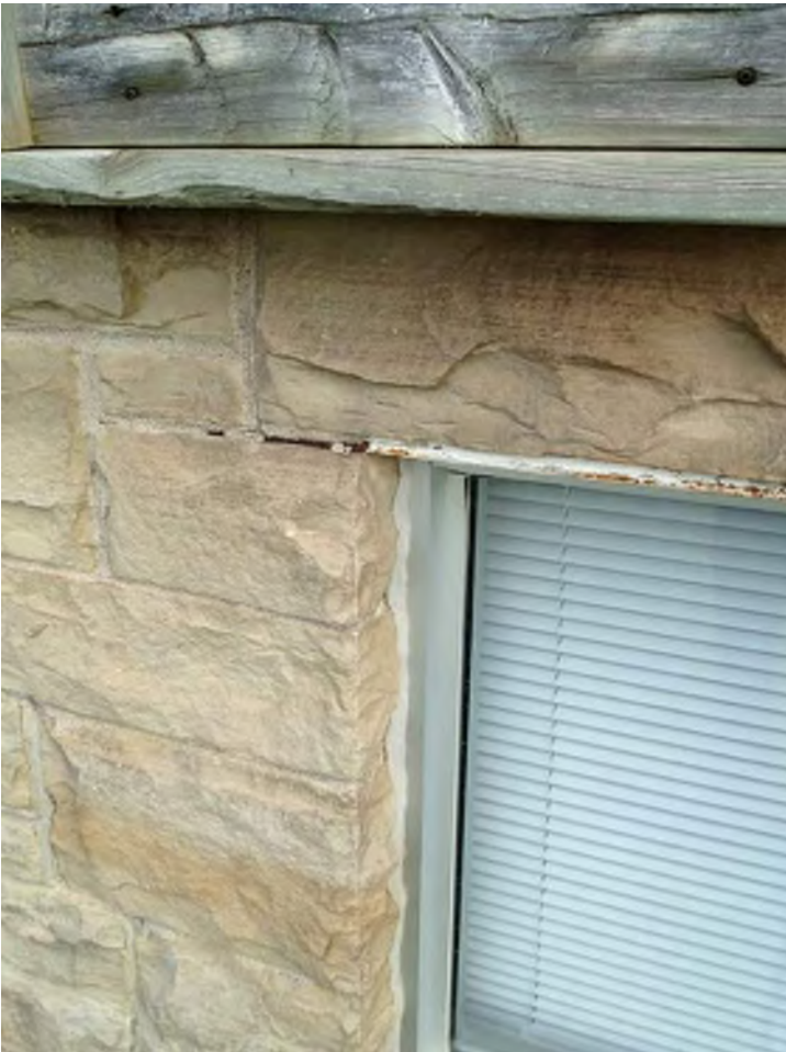
Rusting exterior window lintel and cracked mortar joints.
