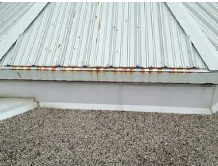
Metal roof over north gymnasium showing rusting
