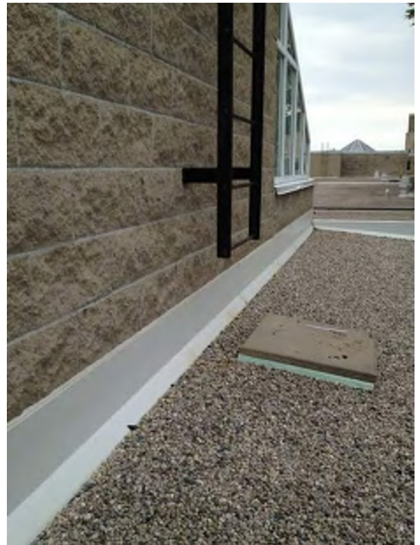
Roof Ladder at 1988 addition - height of bottom rung too high above lower roof.
