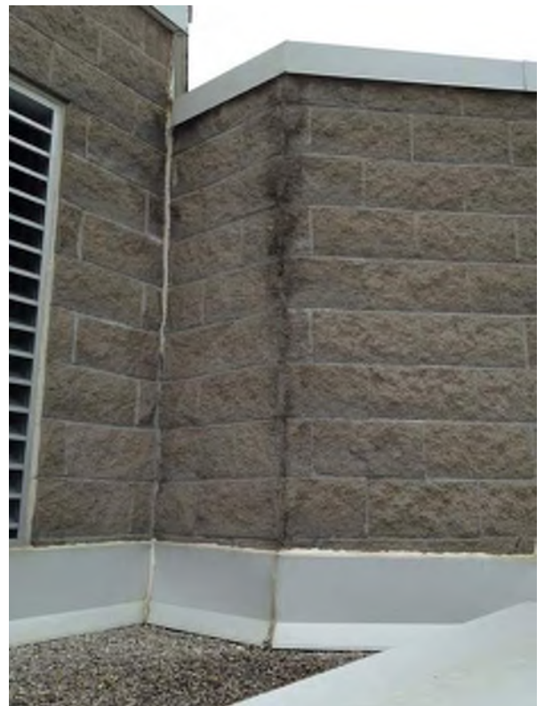
Water damage at concrete block - Upper North Gymnasium Elevation
