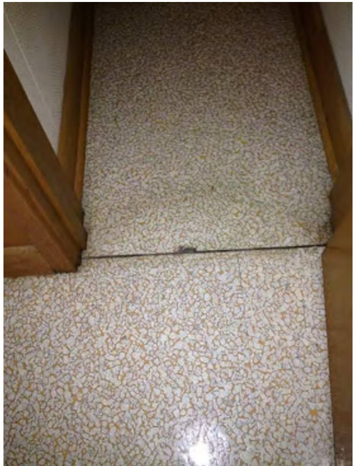
Existing asbestos containing flooring in chapel.
