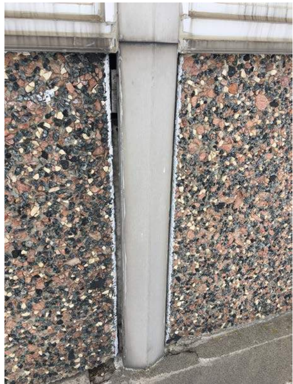
Wall cavity exposed due to gap between precast insulated masonry panels and aluminium cover plate, east elevation of north Y-shaped wing (ERA, 2018).
