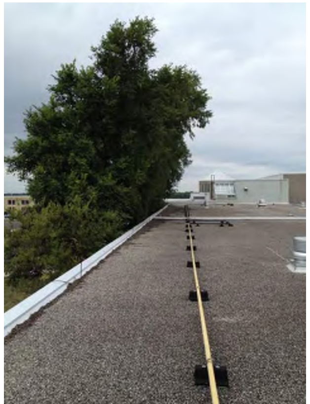
Overhanging trees at Roof H
