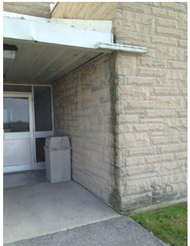
Water damage at eave causing deterioration of mortar joints and staining of stone veneer - 1988 addition
