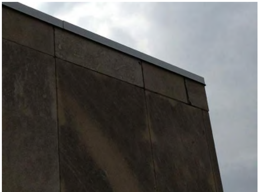
Weathering and deterioration of joints in smooth stone panels on North Elevation.
