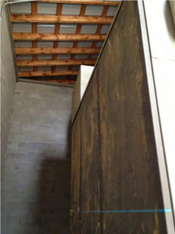
Dust collector enclosure roof - combustible roof construction - not compliant.
