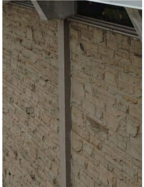
Upper caulking joint at Gymnasium - North Elevation
