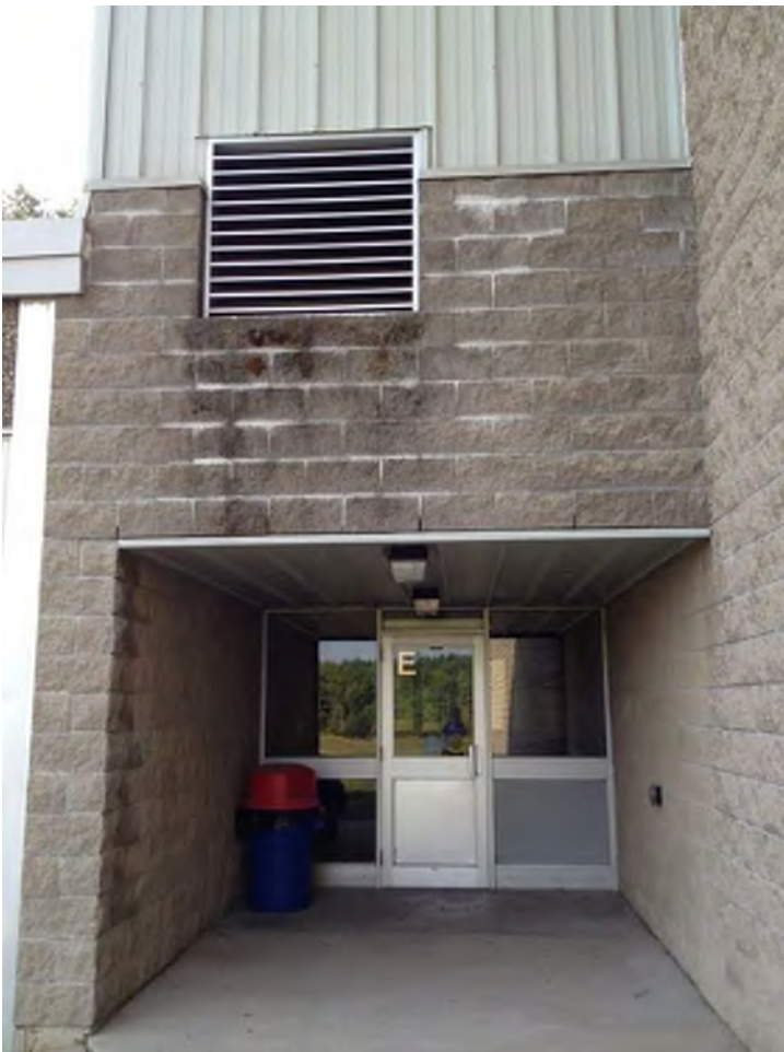
Missing metal sill and flashing at louvre on 1988 addition have caused moisture penetration damaging mortar joints and masonry veneer and growth of moss.
