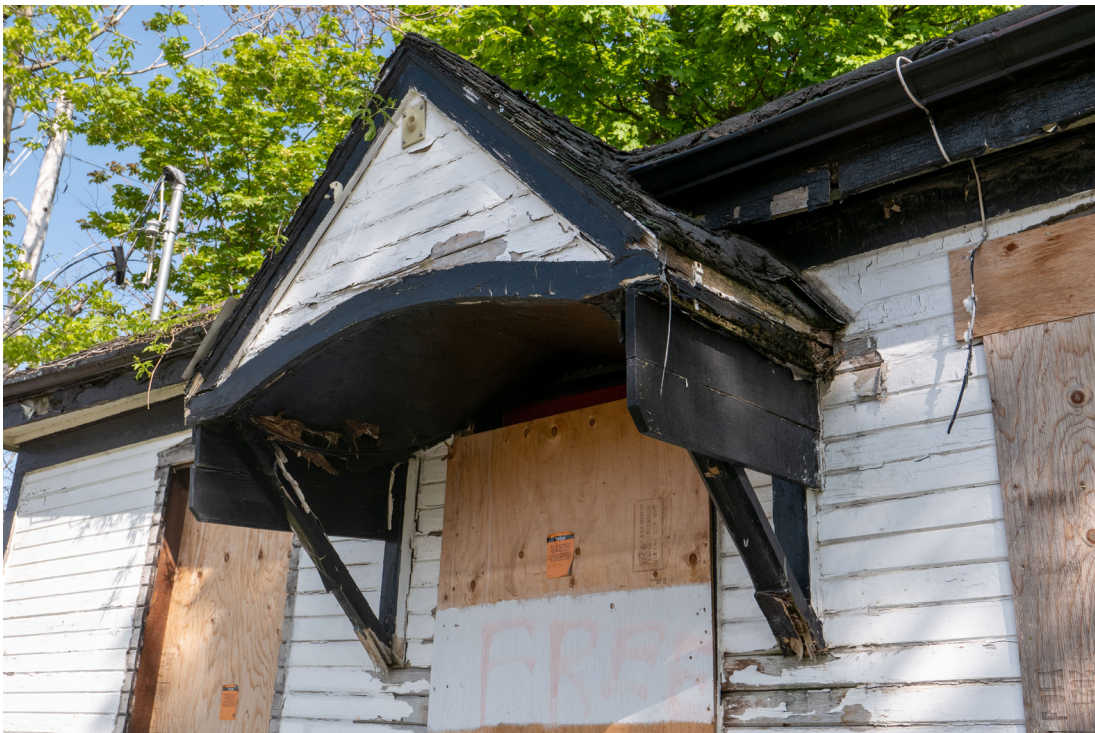
Figure 18: Closeup view of the front porch roof. No major evidence of previous detailing was observed (CBCollective, 2023).
