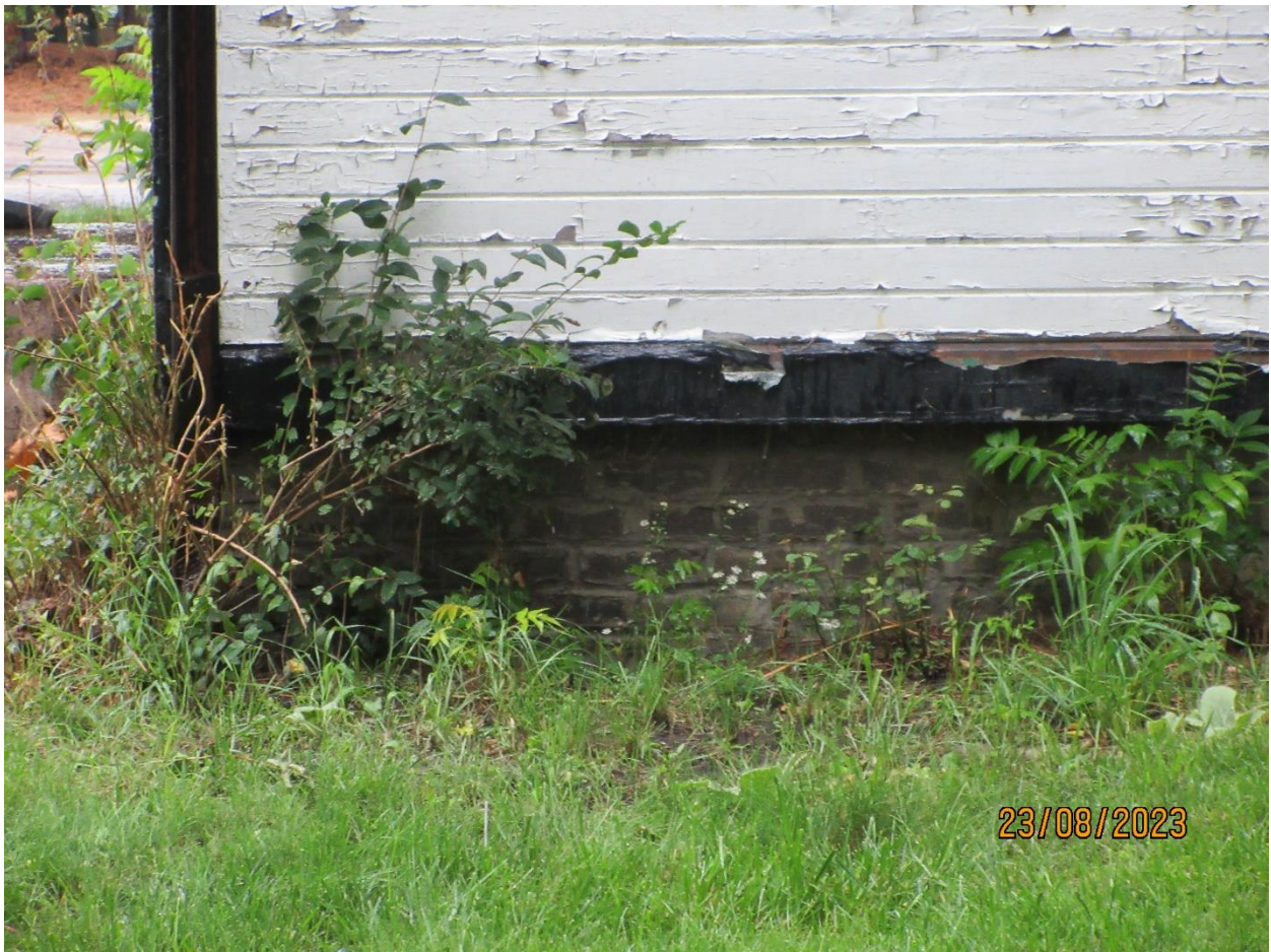
Image 8: Buff brick foundation and peeling paint on wood siding on the east elevation of the building on the subject property at 176 Piccadilly Street, August 23, 2023.
