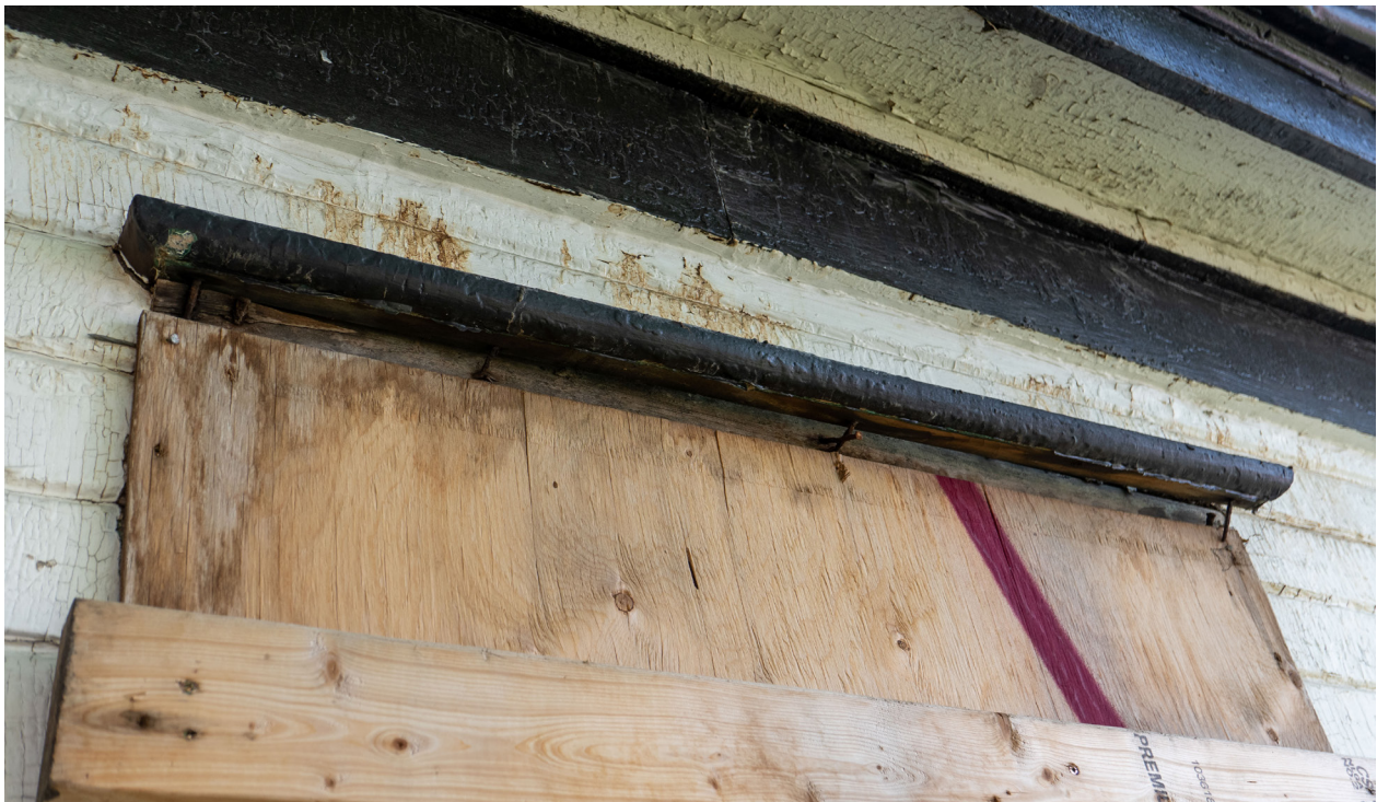
Figure 20: Remnant wooden cornice above the window opening on the west elevation (CBCollective, 2023).
