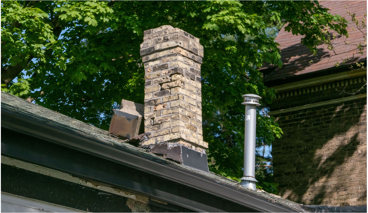
Figure 17: Detail of the chimneys, with former cast chimney cap dislodged and resting against the brick structure (CBCollective, 2023).
