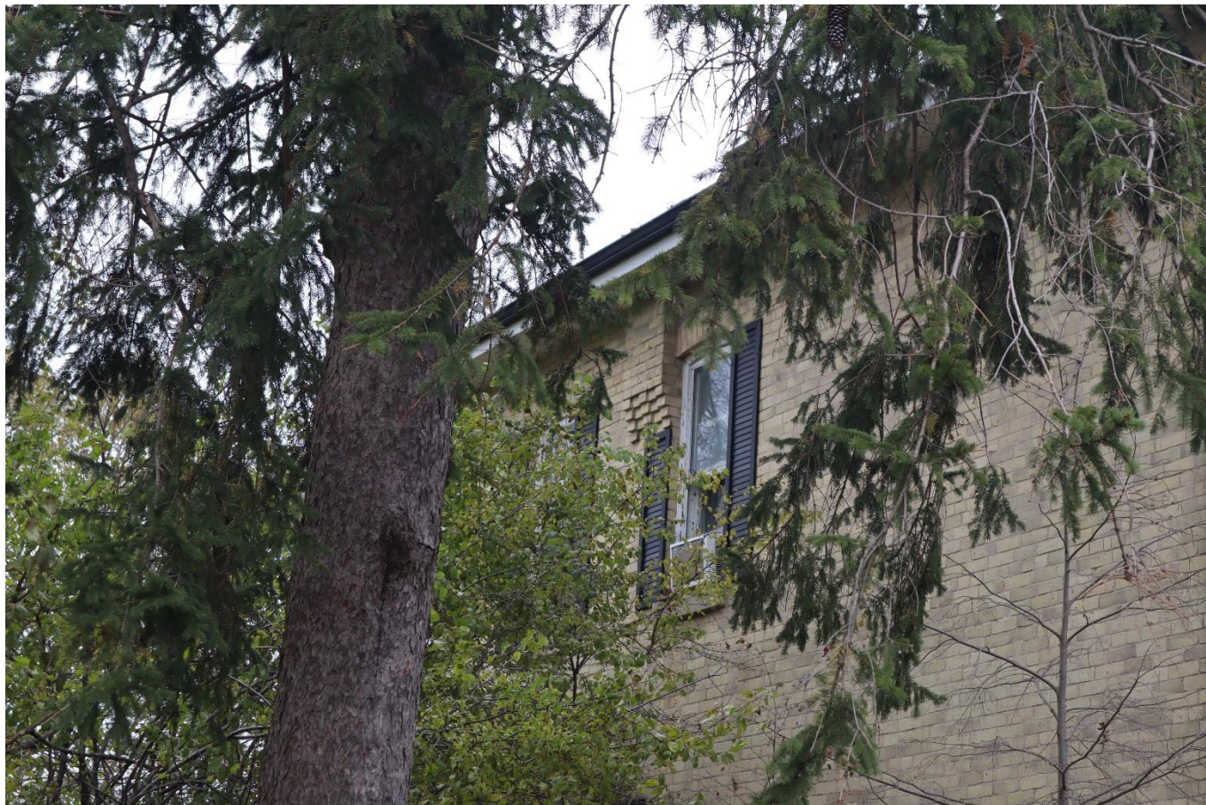
Photograph 16: View of the brick corbelling located on the western elevation, looking northeast (AECOM 2021)
