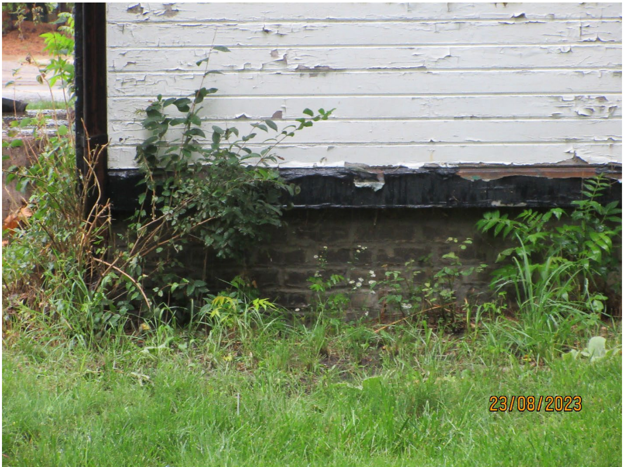
Image 8: Buff brick foundation and peeling paint on wood siding on the east elevation of the building on the subject property at 176 Piccadilly Street, August 23, 2023.
