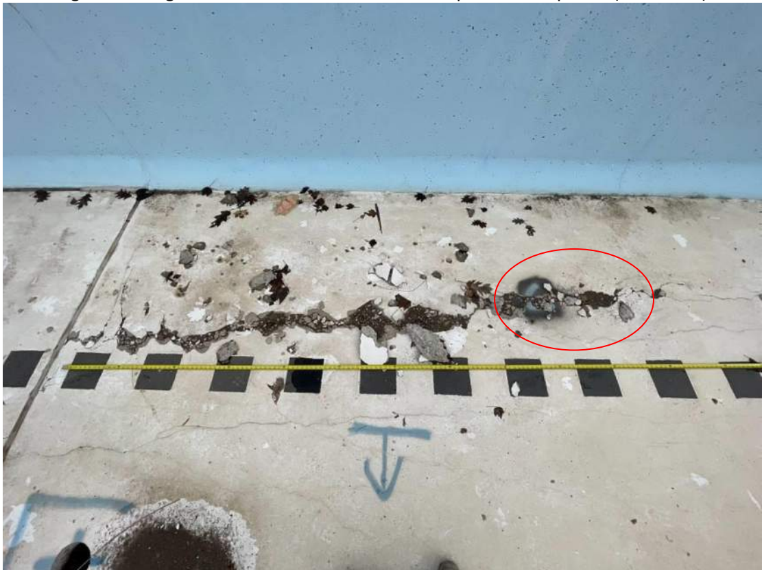
Figure 2b – Significant fracture in lane 1 at break point to deep area (April 2023)
