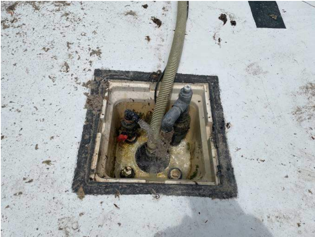
Figure 1 – Ground water in main drain, with pump
