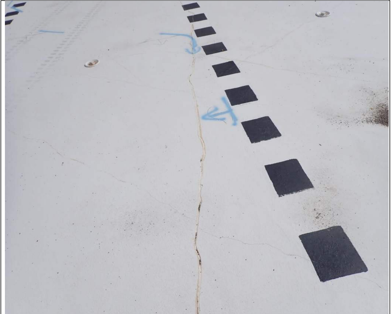
PHOTOGRAPH 8: Large Size Cracks present in the concrete forming pool floor slab.
