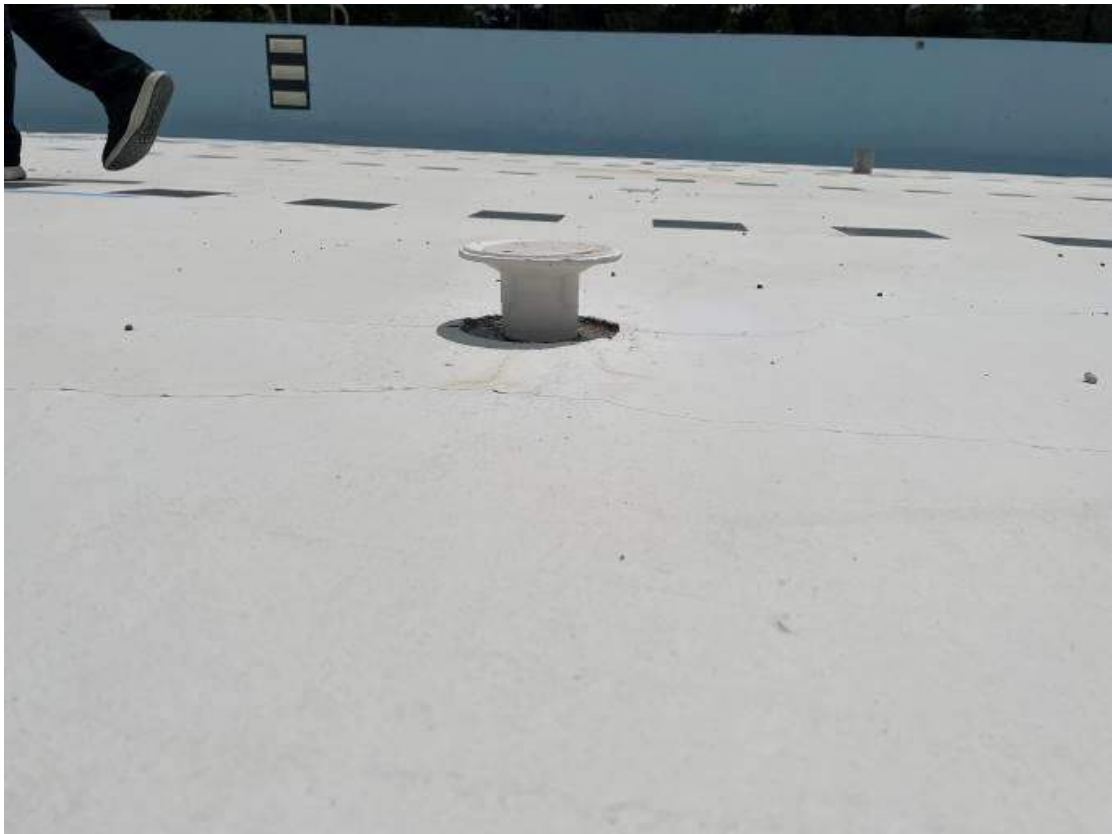
Figure 3 – Floor return protruding from pool floor
