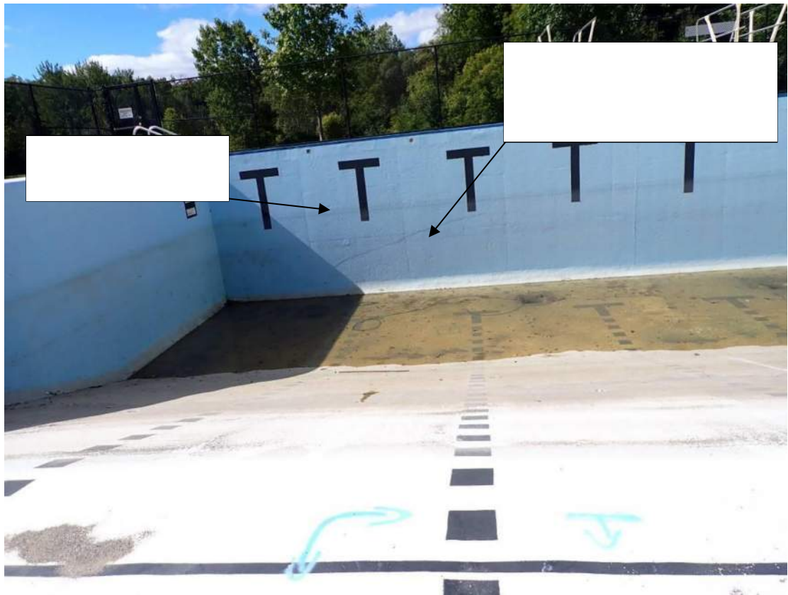
Figure 3b – Debris marking water flood line and lost water line (April 2023)
