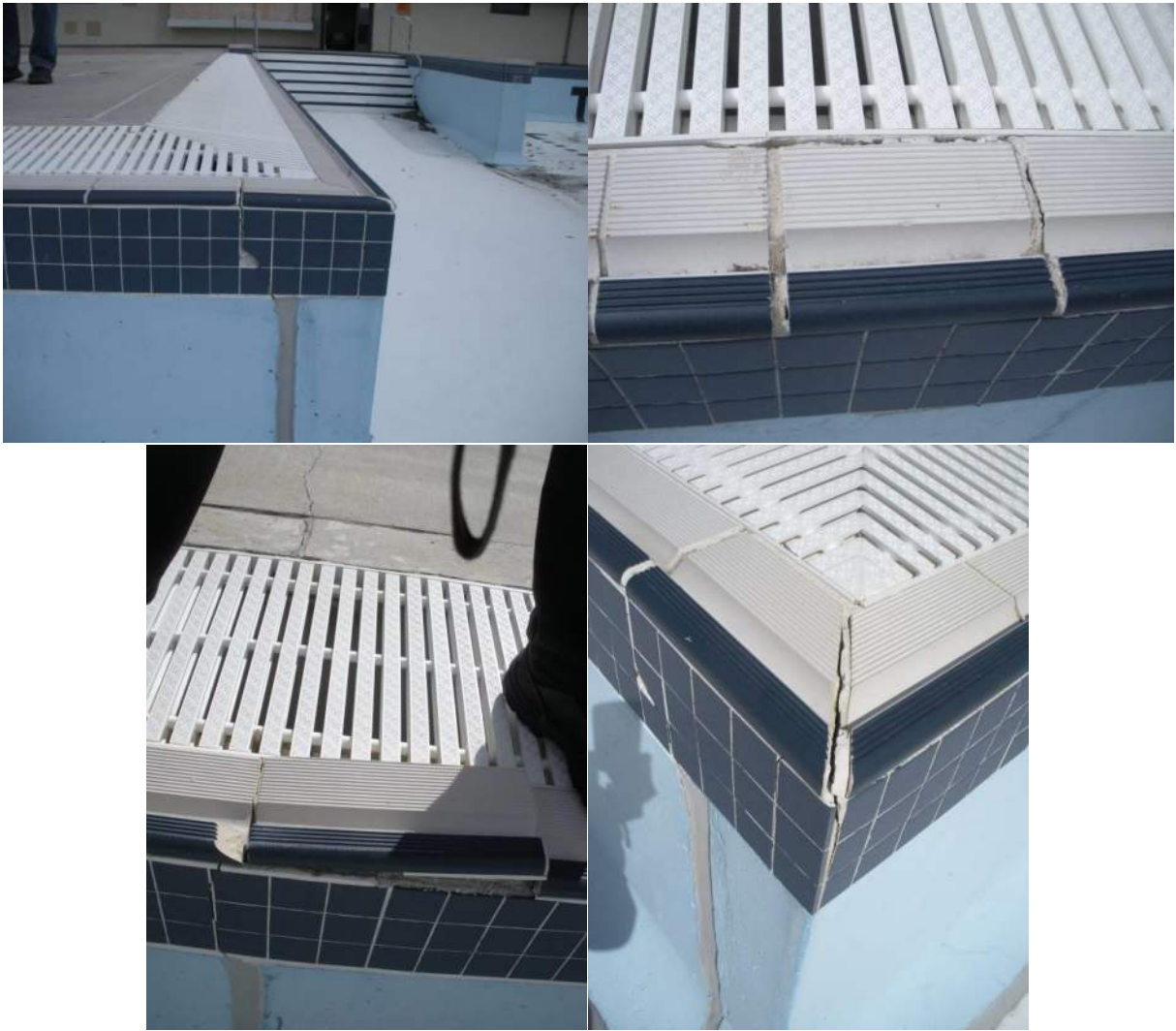
Figure 6 – Original coping damage, prior to recent renovation Indication of pool tank / deck movement (Photos from 2016)
