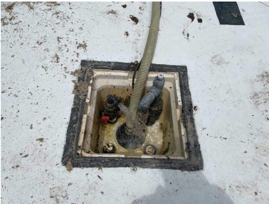
Report I - Ground water in main drain, with pump, June 2022
