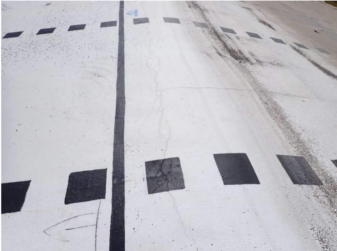
Figure 5a – Cracking at deep-end slope point (September 2022)
