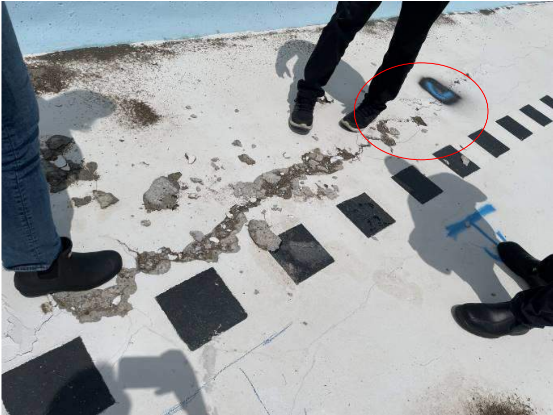
Figure 2a – Significant fracture in lane 1 at break point to deep area (June 2022)
