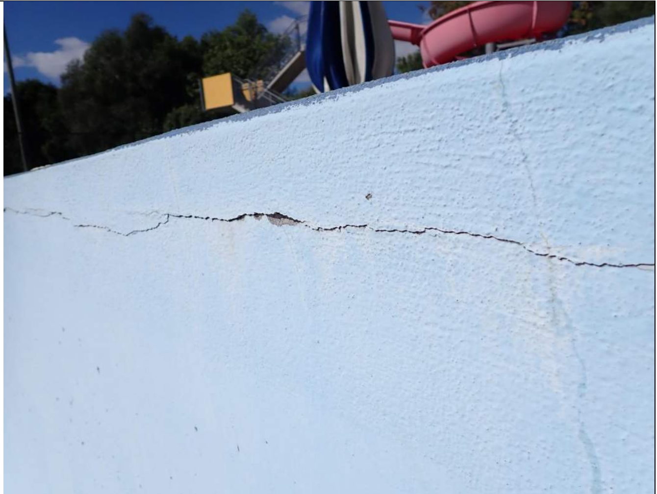
PHOTOGRAPH 11: Longitudinal cracking of the concrete forming pool wall
