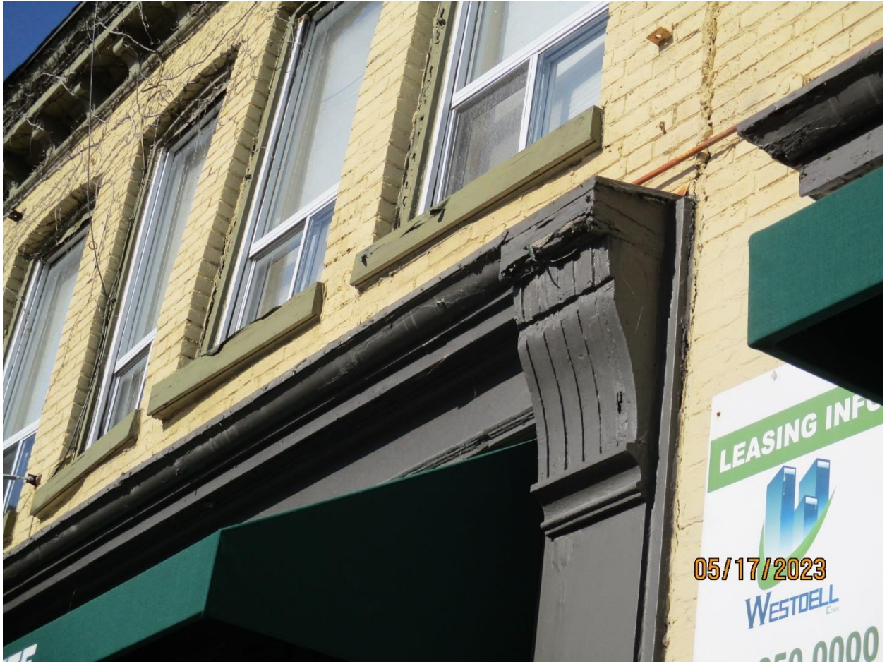
Image 3: Photograph showing corbel and cornice details above storefront on the building at 599 Richmond Street.
