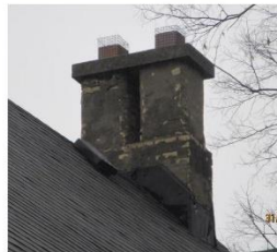
5. Chimney on the north gable, originally paired with a chimney on the south gable (not extant)
